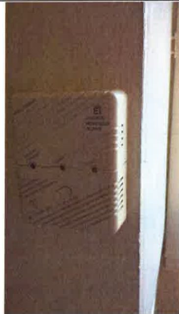
CO Detector Living Room adjacent to Boiler
