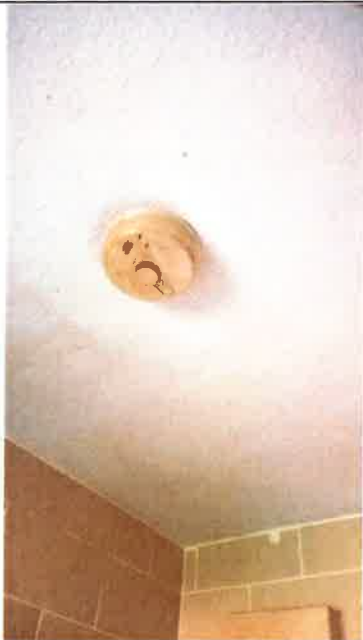
Hard Wired Heat Sensor in kitchen
