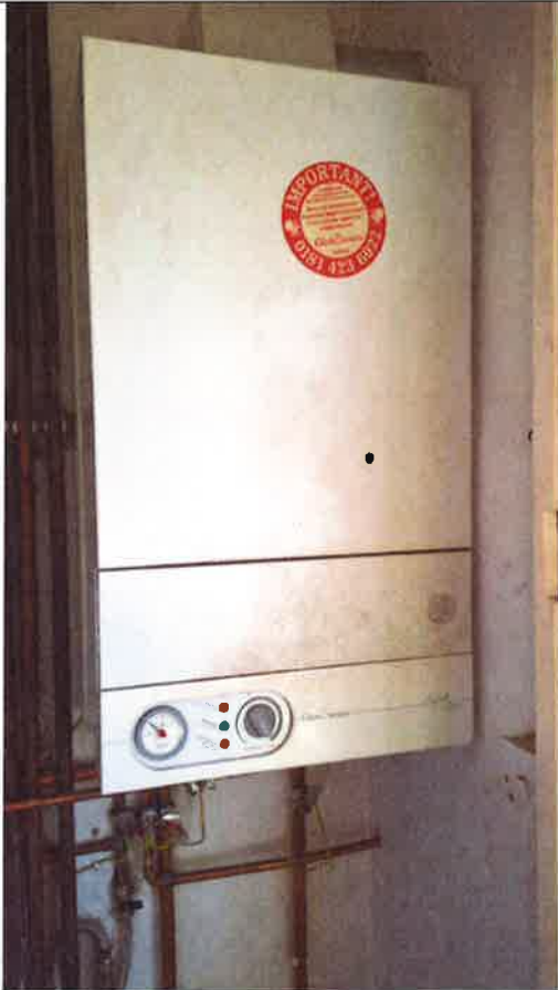
Boiler. Confirmation required that it has been inspected and is in good working order.
