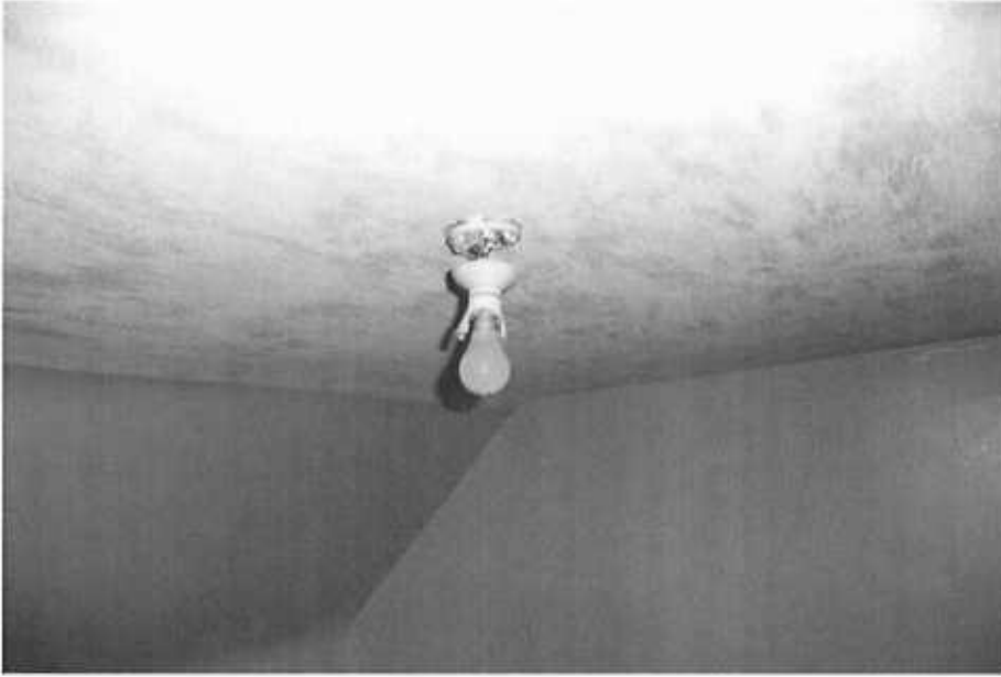
Loose light fitting on 1 st floor
