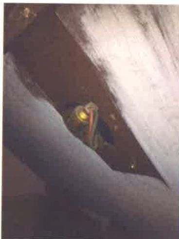
Light fitting roofspace
