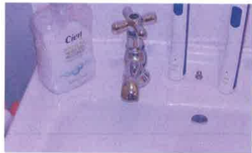
Photo 5 – Defective tap on basin
