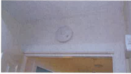
Photo 8 – Heat + Carbon Monoxide alarms
