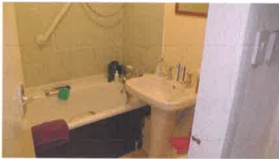
Photo 4 – Pedestal wash hand basin
