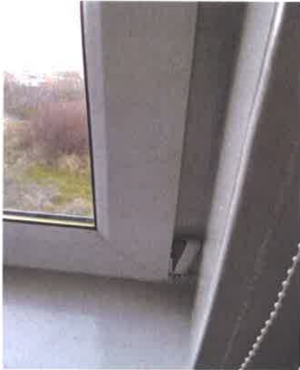
Photo 2 – Damaged window hinge in Bedroom
