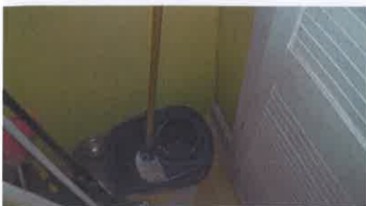
Photo 7 – Saturated wall section
