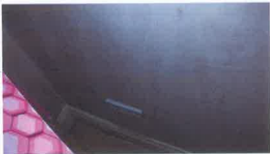
Photo 11 – Hole at socket
