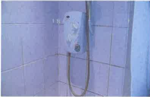
Photo 5 – Embedded damp in wall
