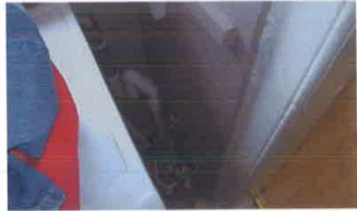
Photo 10 – Saturated wall section
