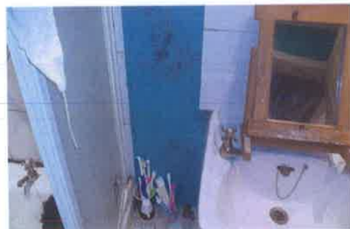
Photo 4 – Saturated wall section
