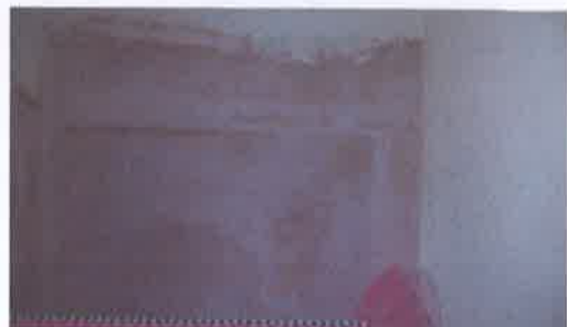
Photo 8 – Damp wall section
