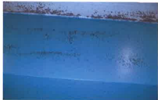
Photo 6 Embedded damp in beam
