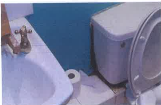
Photo 3 – Saturated wall section
