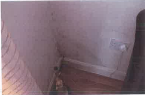
Photo 1 – Saturated wall section
