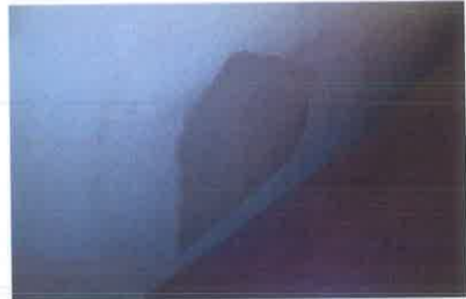
Photo 2 – Saturated wall section
