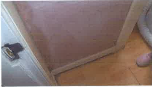
Photo 9 – Saturated wall section
