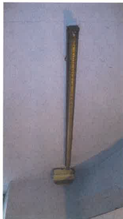
Photo 7 – Long defunct kitchen strip light
