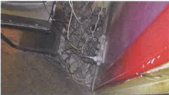
Photo 14 – Tangle of wiring, leads and extension cables
