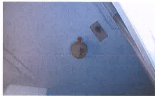
Photo 11 – Defunct smoke detector in hall way
