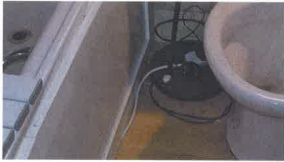
Photo 16 – Inappropriate power supply to bathroom
