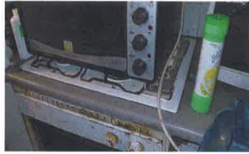
Photo 9 – Non serviceable gas hob above oven
