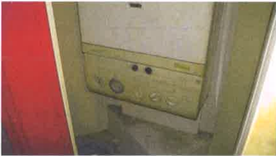
Photo 12 – Gas boiler in living room cupboard
