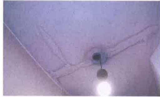
Photo 3 – Exposed wires + water staining in hall
