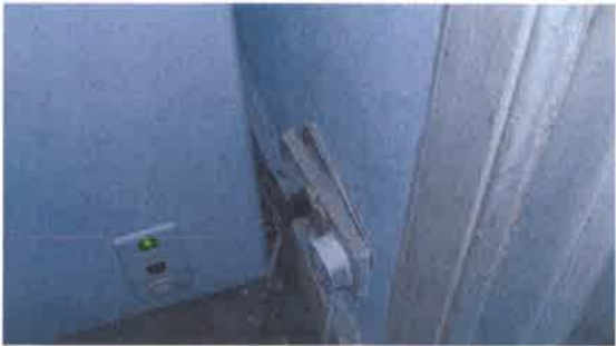
Photo 4 – Damaged double socket in hallway
