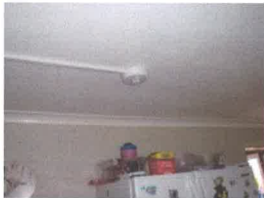
HEAT DETECTOR – KITCHEN
