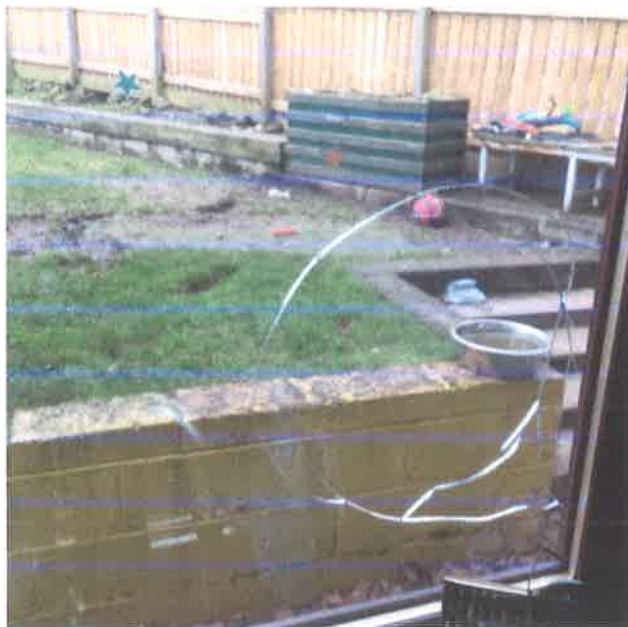
4. Broken glazing unit - kitchen
