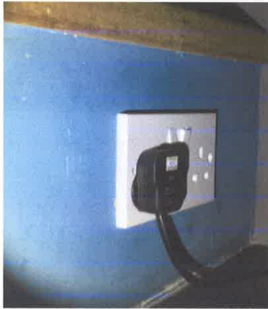
7. Replacement double socket at worktop
