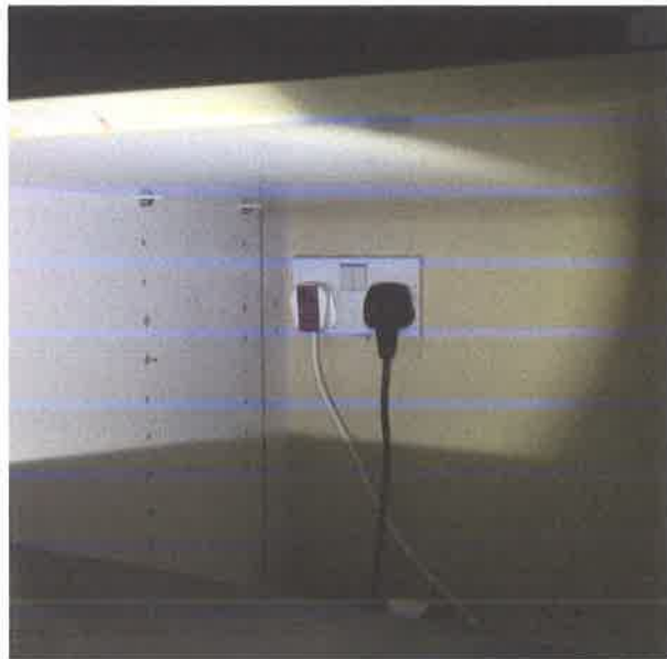
6. Wiring arrangement behind oven
