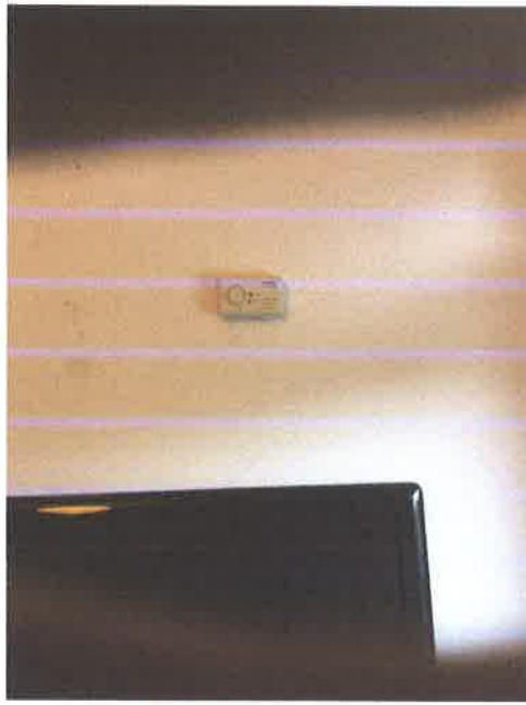
13. Carbon Monoxide detector front bedroom
