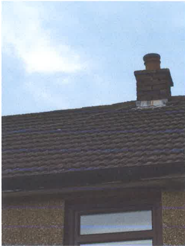
3. Cracked mortar at ridge
