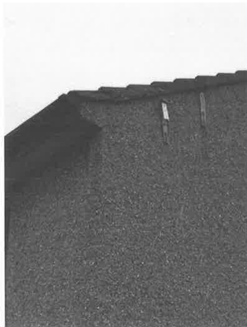
2. Cracked tifting at verge
