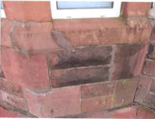
Front elevation - stonework recently re-pointed under living room bay window
