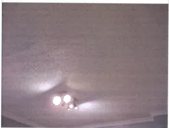
Kitchen - no heat alarm
