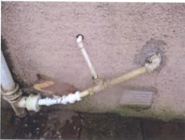
Rear elevation - waste pipe from bathroom - external roughcast to surrounding wall patched
