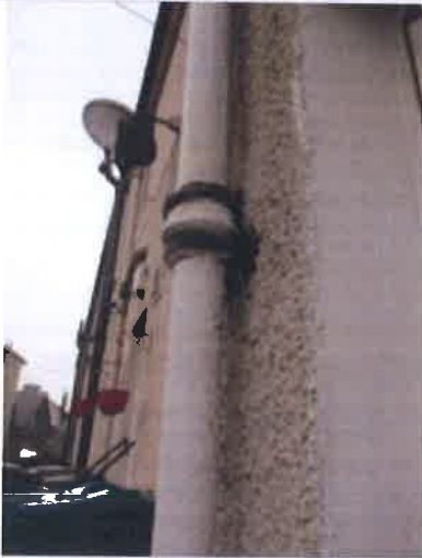
Rear elevation - soil pipe defective and not secured to wall properly
