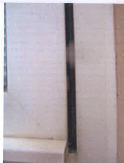
Front bedroom - external view - defective window/mechanisms - large gap to side
