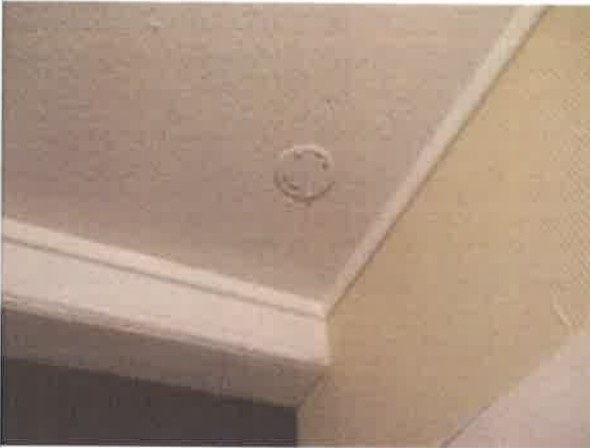
Hall - ceiling mounted fitting/smoke alarm missing
