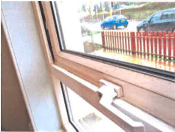
Front bedroom - internal view - defective left side window - sealed shut
