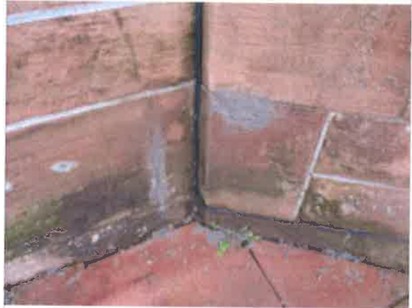
Front elevation - stonework recently re-pointed under and to side of living room bay window
