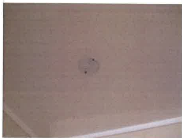
Hall - 2nd ceiling mounted fitting/smoke alarm missing
