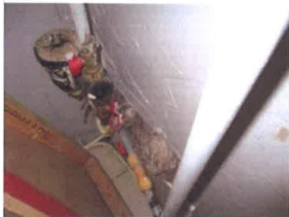
Kitchen - pipes and wiring exposed under boiler
