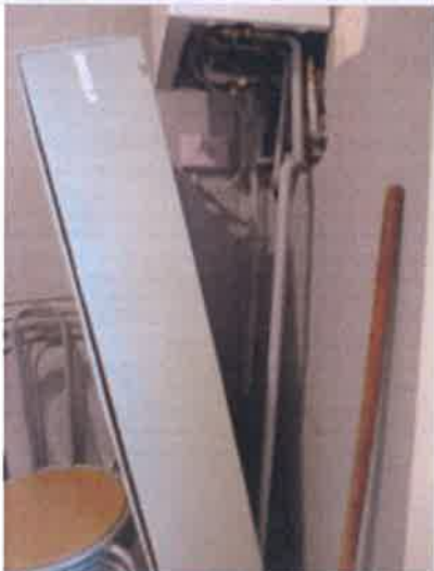
Kitchen - pipes and wiring exposed under boiler, defective/loose boxing
