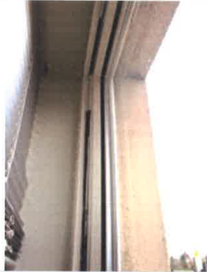
Front bedroom - internal view - defective left side window damaged seals
