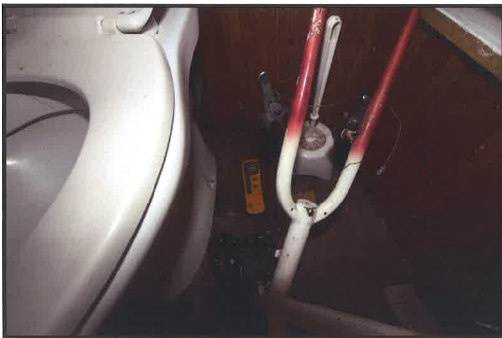
Figure 14 Bathroom floor and meter reading.
