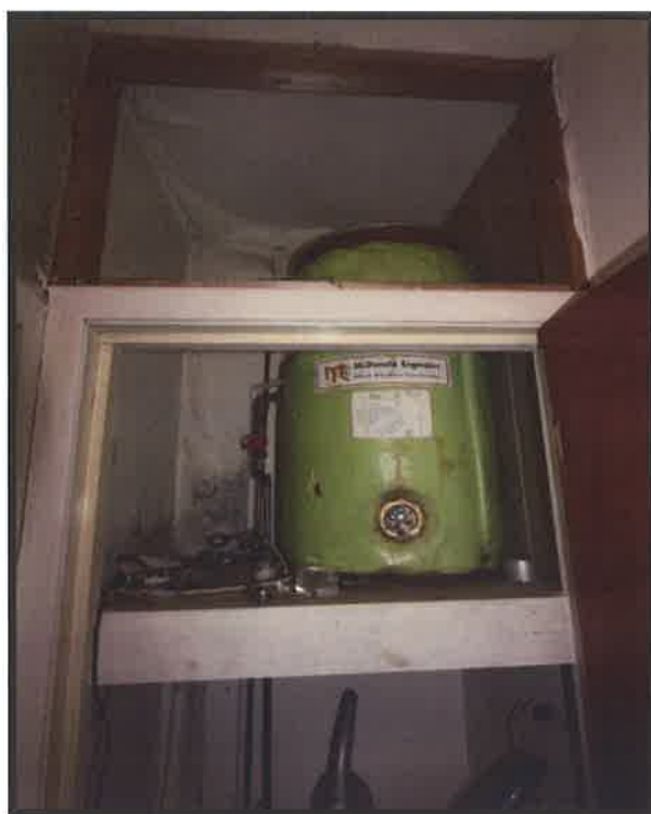
Figure 8- Airing cupboard/immersion heater.
