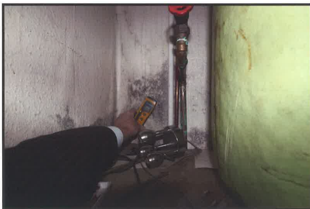
Figure 9 Mould to walls, airing cupboard.
