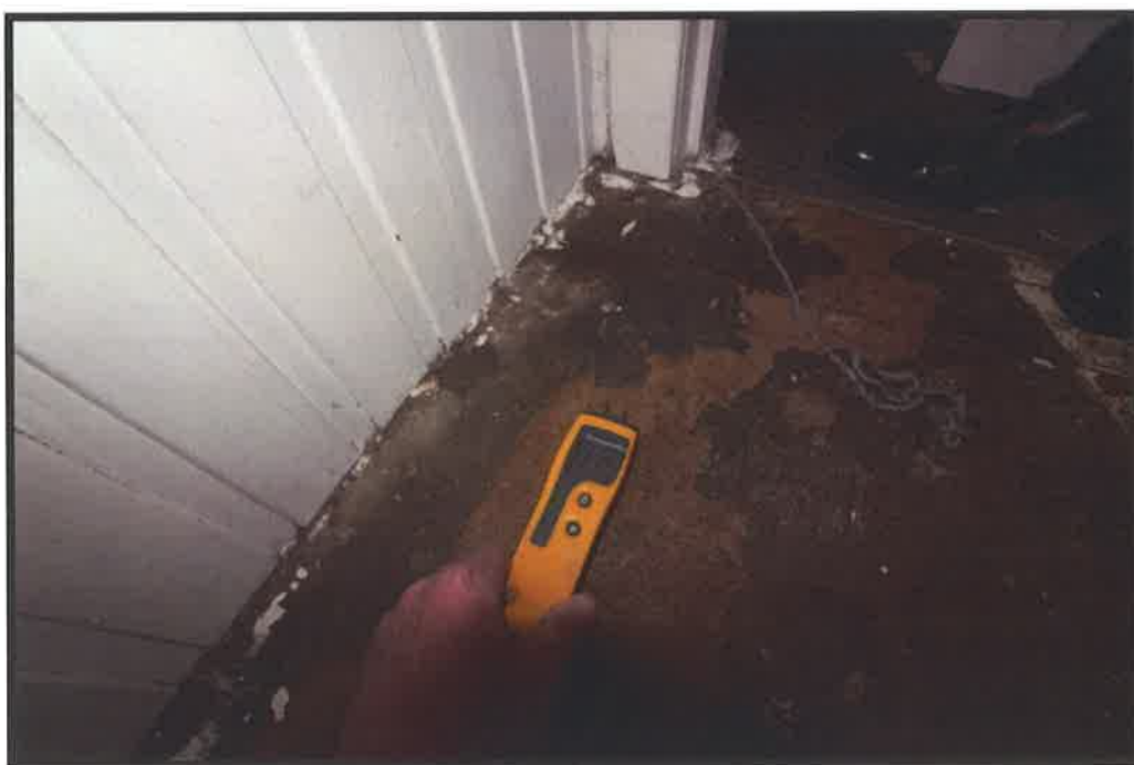
Figure 13 Bathroom floor and meter reading.
