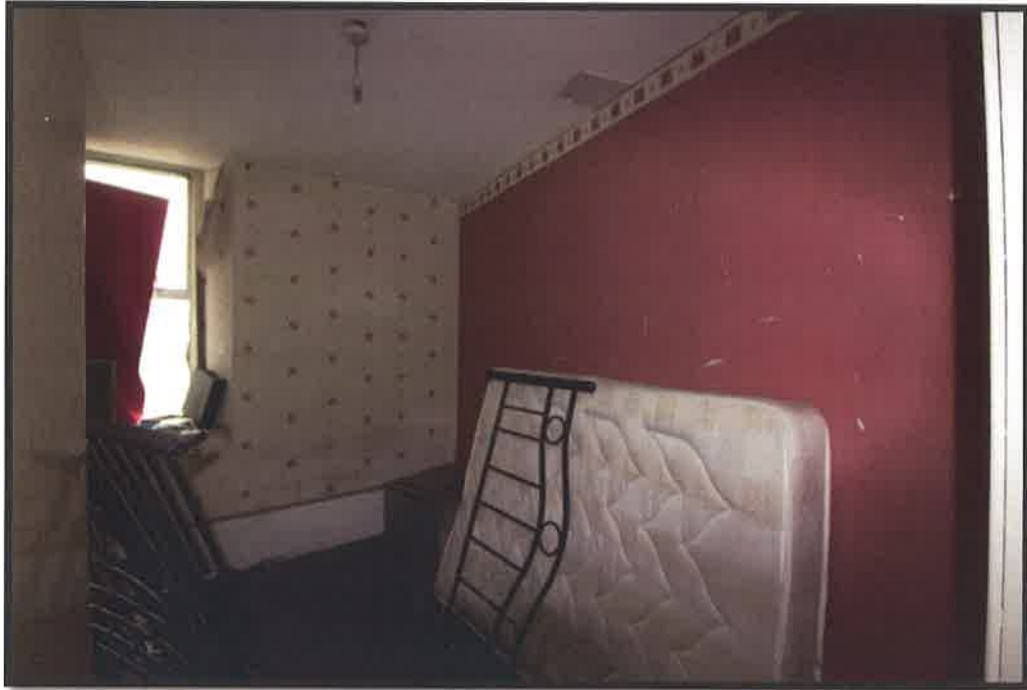
Figure 10 Bedroom overview - loose ceiling rose, patched ceiling.
