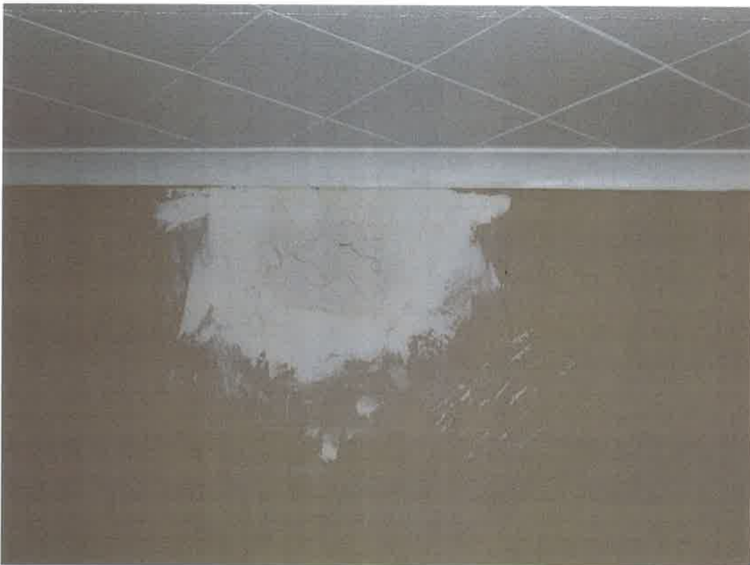
Living room wall – damaged plaster finish at high level – cause unknown.
