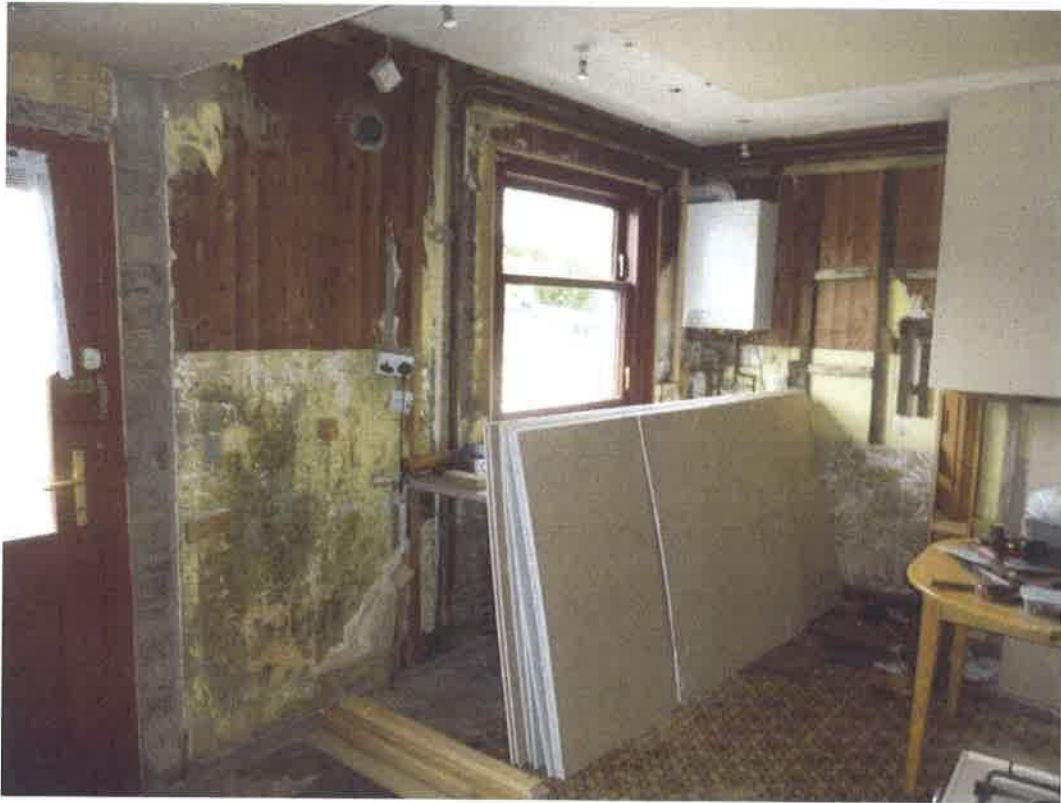
Kitchen – general view showing no wall linings and poor floor
