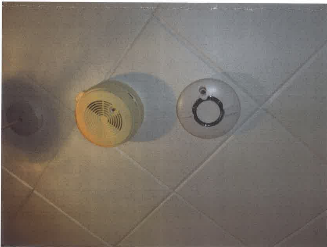
Top landing – old hard wired mains smoke detector adjacent to newer linked smoke detector
