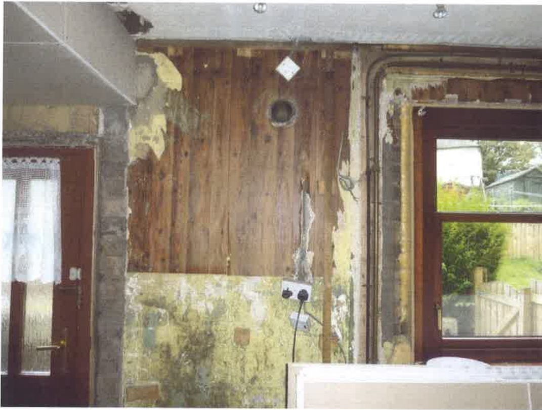
Kitchen – poor electrical installation and no wall lining
