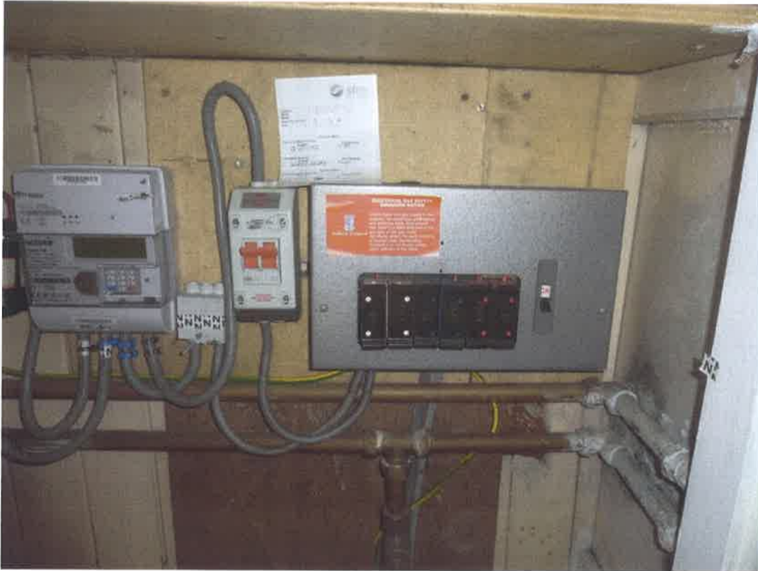
Mains electrical distribution board – requires updating or replacing with appropriate board and EICR
