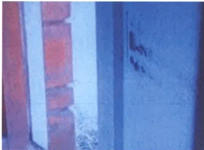
7:- Damaged internal wall plaster caused by ill fitting living room door
