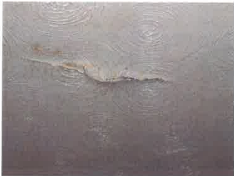
4:- Damaged kitchen ceiling plaster
