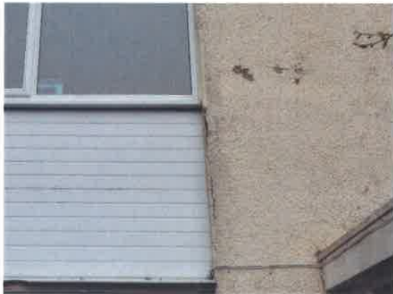
8:- Defective rendering front wall
