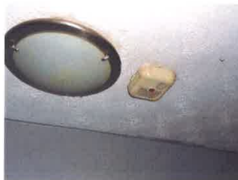
5:- Broken / defective battery operated smoke alarm on landing ceiling
