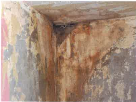
2:- Defective wall plaster in rear bedroom
