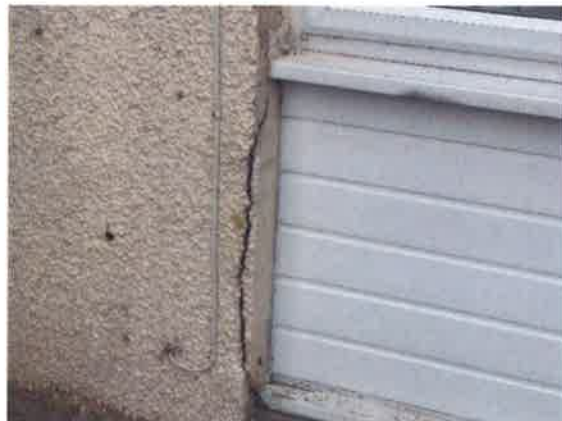
9:- Defective rendering front wall
