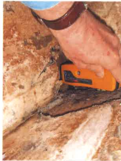
3:- Damp readings (23%) in rear bedroom external wall
