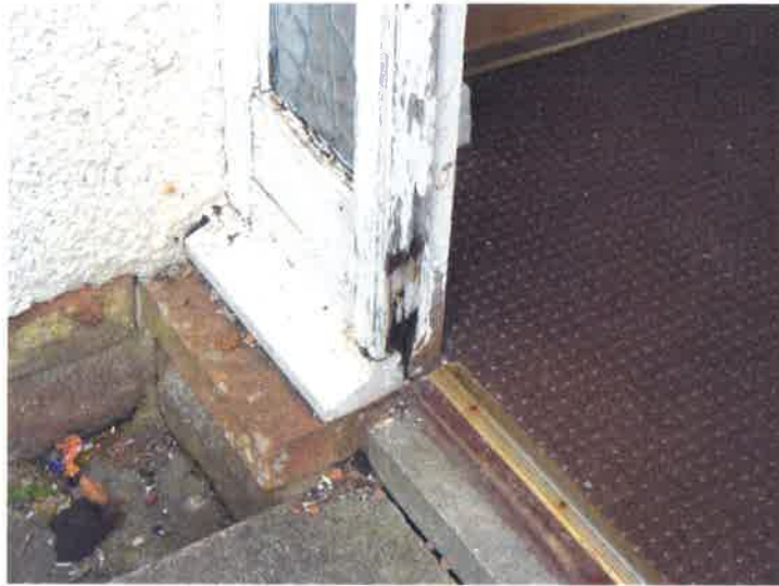
6:- Rotted external timber frame at front entrance door
