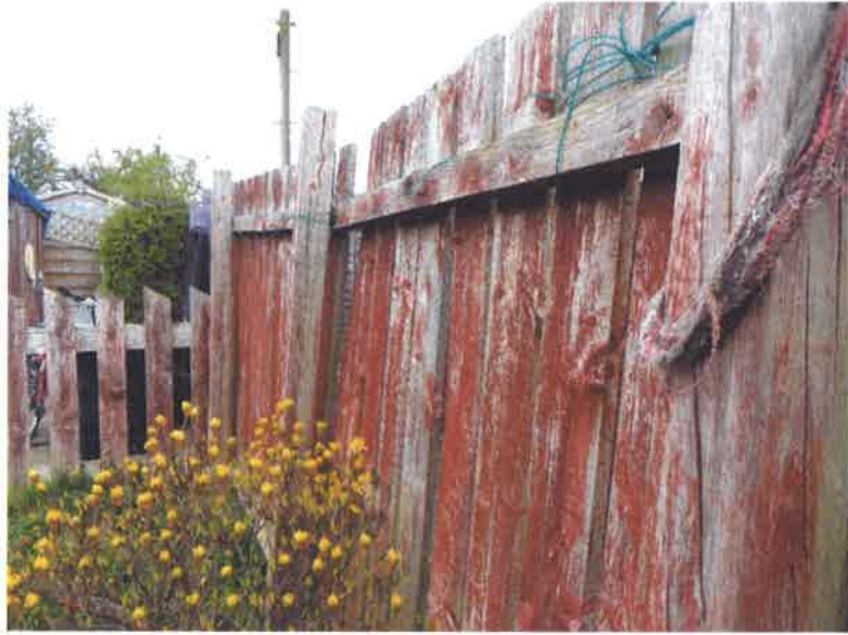
10:- Broken rear fence from garden
