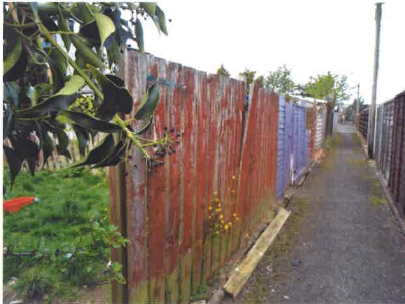
11:- Broken rear fence from rear path
