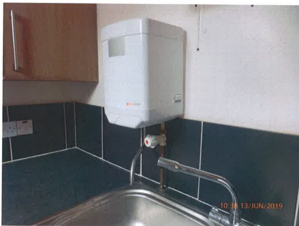
Hot water heater in the kitchen
