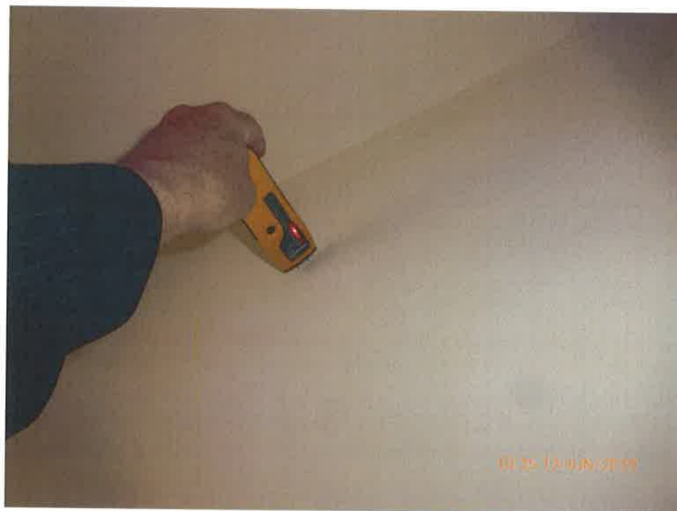
Dampness in bedroom below the stack
