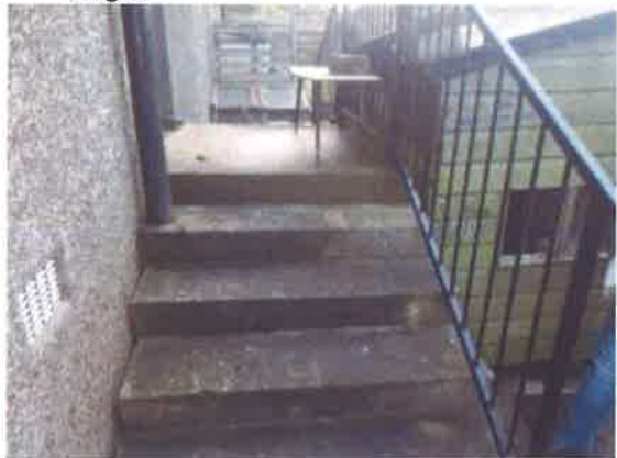
30 Rear entrance steps – loose.
