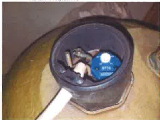
12 Unsecured cap to cylinder.
