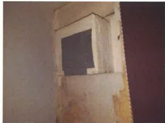
26 Extract ventilation blocked.
