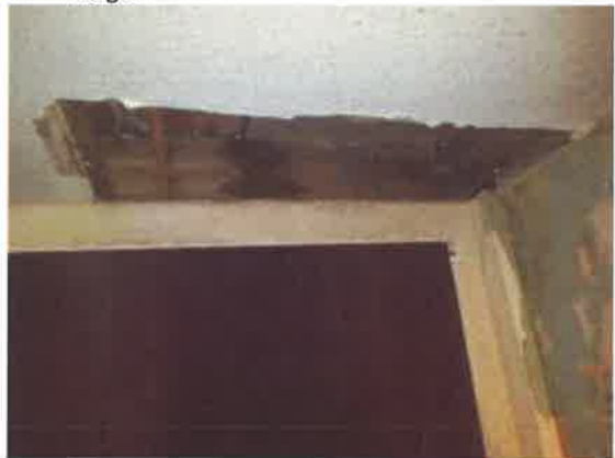
22 Ceiling damage remains.
