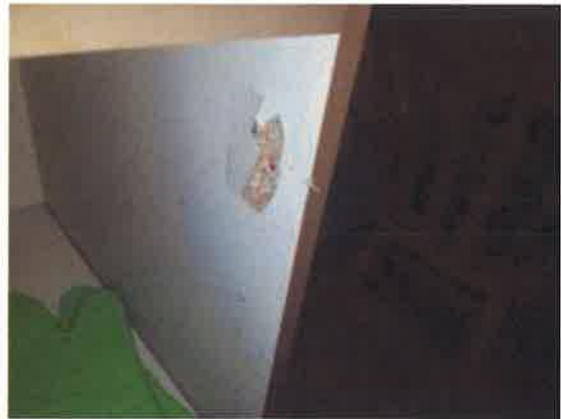
20 Damage to base unit in kitchen.
