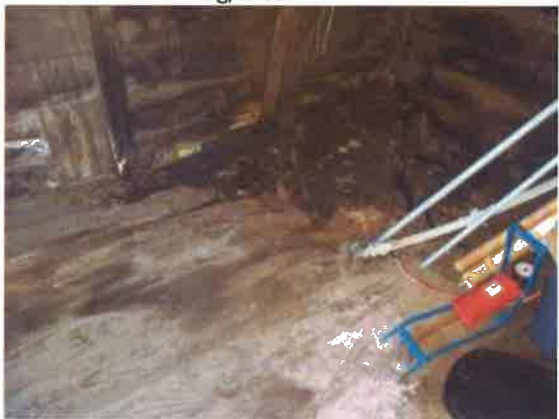
42 Timber decay to floor of shed and framework.
