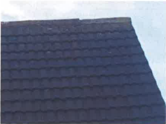
29 Damage at ridge.
