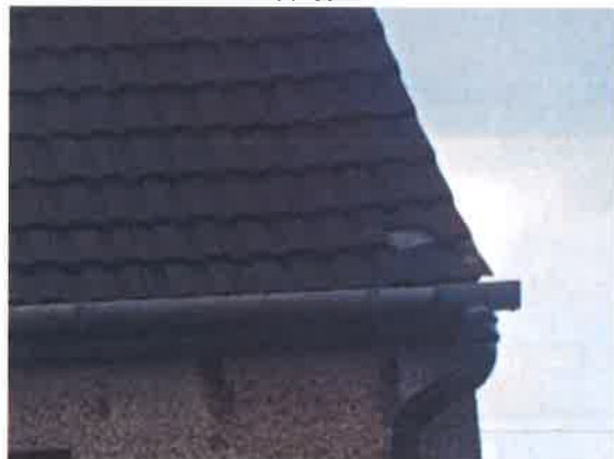
28 Damaged roof tiles.
