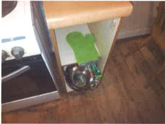
19 Kitchen base unit – doorfront missing.
