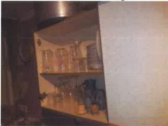
21 Missing doorfront to wall unit.
