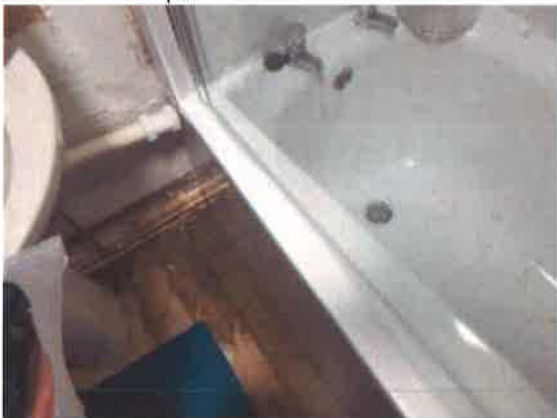
9 Water escape adjacent to bath.
