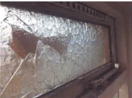
5 Cracked glass to top hopper - bathroom.
