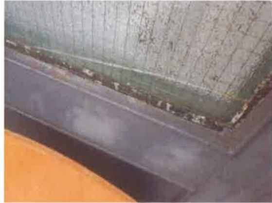
2 Cracked side glazed entrance panel.
