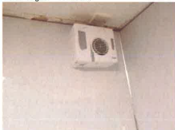
6 Extract ventilation - bathroom.
