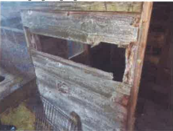
41 Damage to external paneling to shed.
