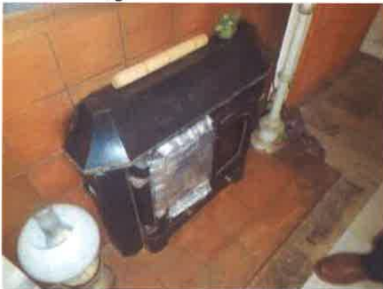
48 Fire within Living Room.
