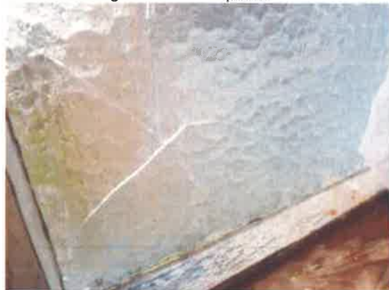
4 Cracked glass - bathroom.
