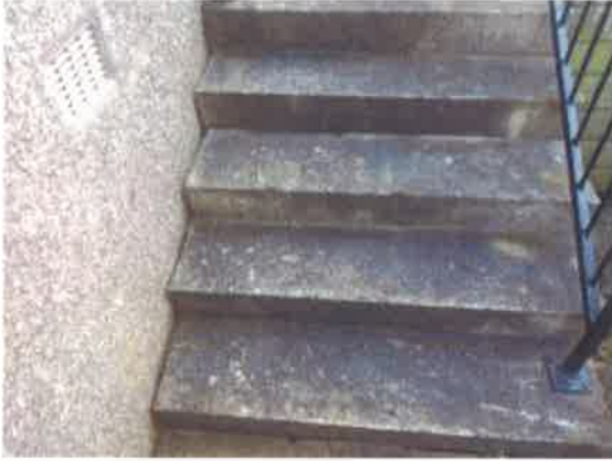
37 Rear steps – loose.
