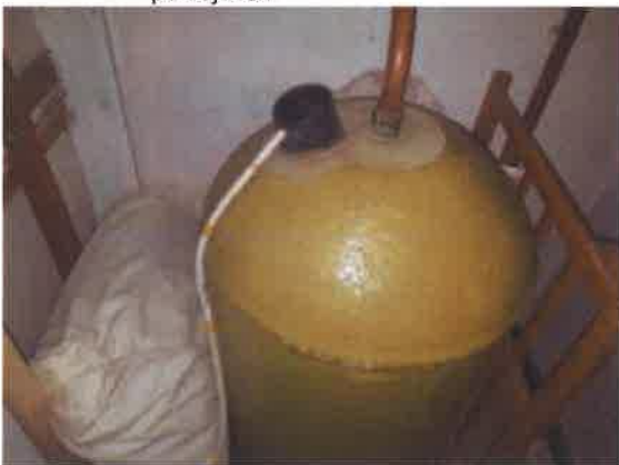
11 Hot water cylinder.
