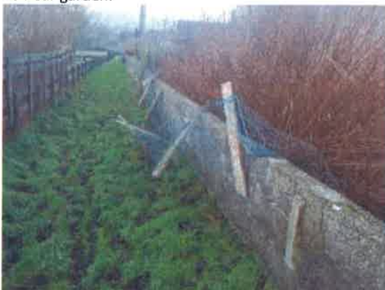
45 Fencing failed to boundary wall.
