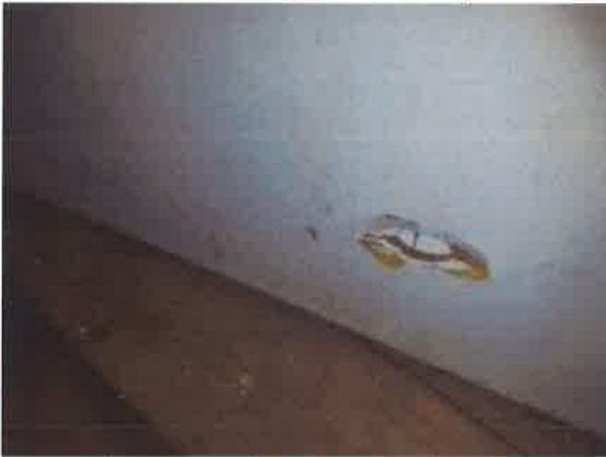
15 Example of impact damage to pass door.
