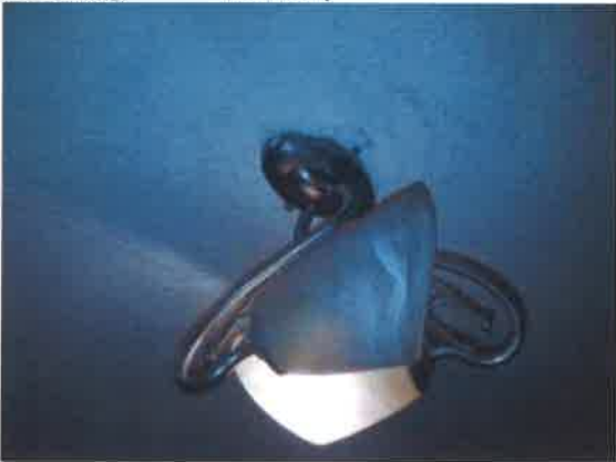
47 Light fitting defective to Living Room.
