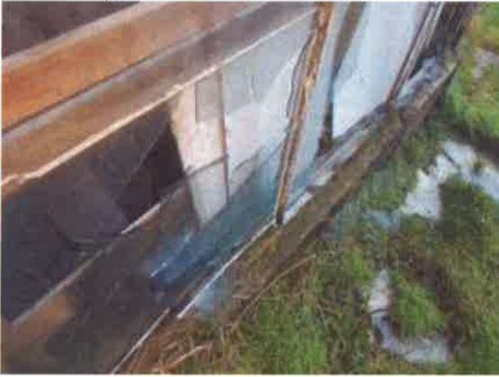
39 Damaged glazing to greenhouse.
