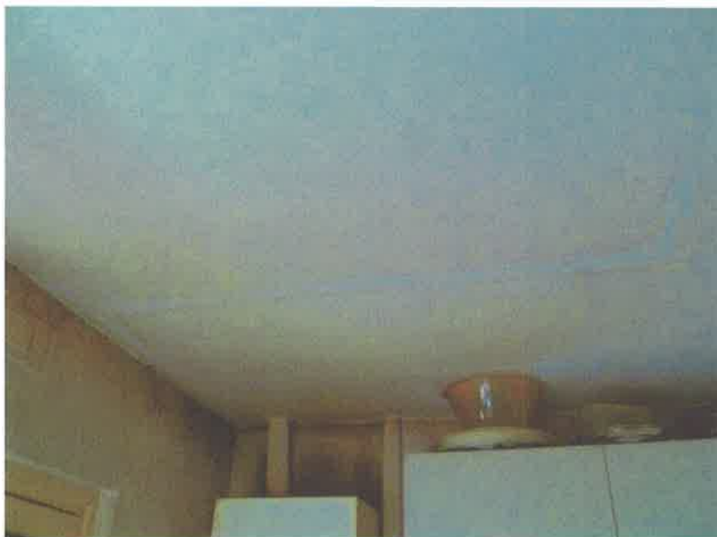
12. Water staining on kitchen ceiling
