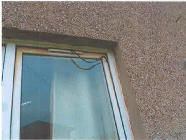
6. Living room rear window showing broken seal
