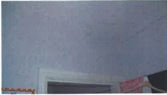
Photo 14 - Kitchen heat sensor
