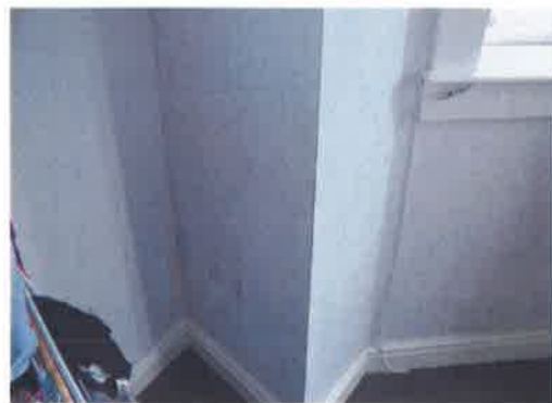
Photo 3 - Dampness in Living Room
