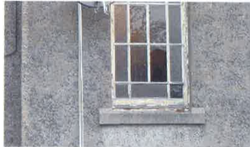
Photo 11 - Missing glass on stairwell
