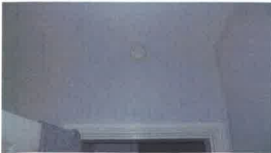
Photo 12 - Living room smoke detector
