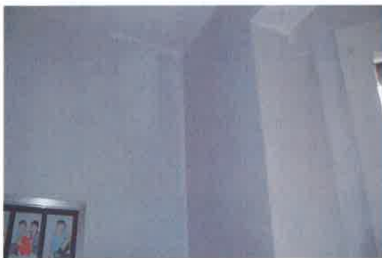
Photo 2 - Dampness in Living Room
