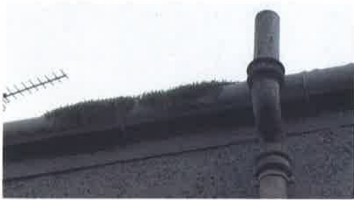
Photo 8 - Blocked gutters on rear elevation
