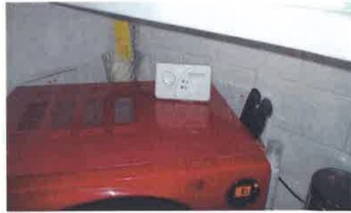
Photo 15 - Carbon monoxide detector
