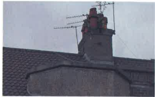
Photo 9 - Chimney head in poor order
