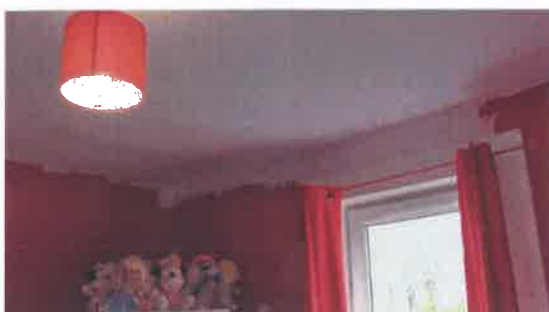
Photo 4 - Evidence of former water ingress
