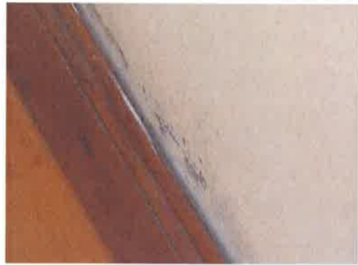
Photo 3 - Mould on bedroom wall
