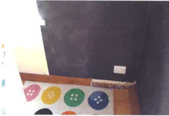
Photo 2 - Light damp levels in bedroom
