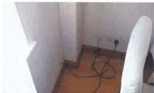
Photo 5 - Dampness in Living Rm.
