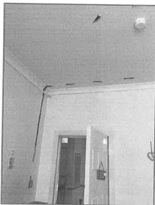
Photograph 3: Channels to ceiling and wall
