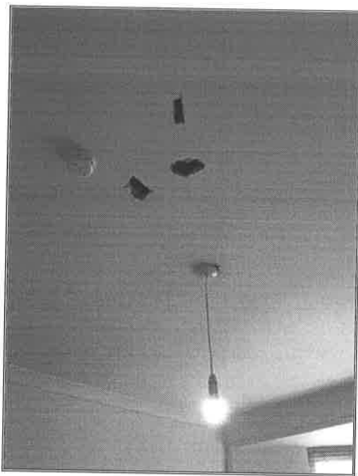
Photograph 2: Holes in ceiling and working pendant light
