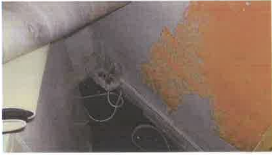
Photo 9 – Damaged socket (Kitchen)
