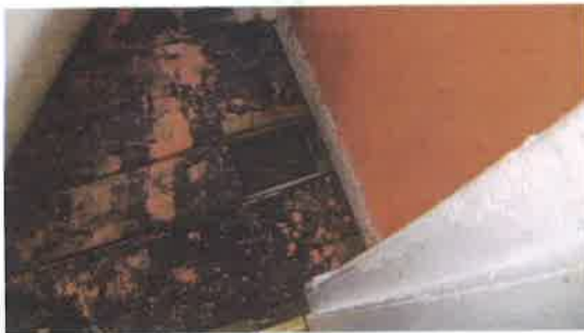
Photo 5 – Damaged kitchen floor
