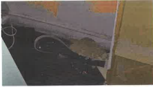
Photo 2 – Rodent access in kitchen
