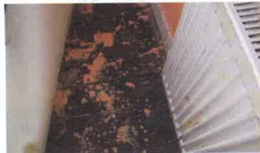
Photo 6 – Damaged kitchen floor
