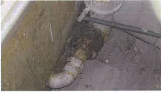
Photo 17 – Rusty waste water pipe
