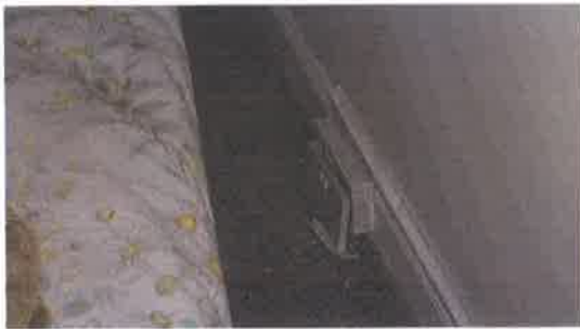
Photo 13 - Damaged socket (Bedroom)
