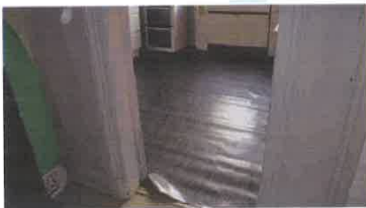
Photo 7 – Damaged kitchen linoleum
