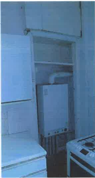
Photo 19 – Boiler in kitchen
