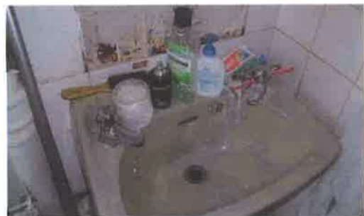
Photo 16 Missing tiles/leaking tap
