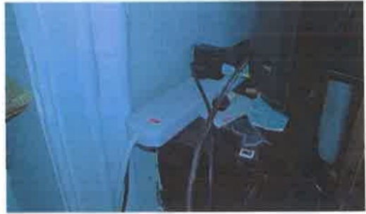
Photo 10 - Ext. cable in living room
