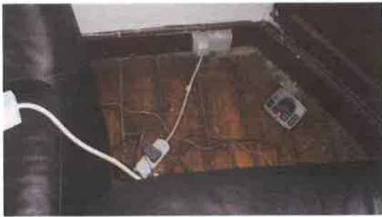
Photo 11 - Ext. cables in living room
