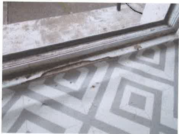
Kitchen - new vinyl floor covering - poor fitting - trip hazard at threshold to back door
