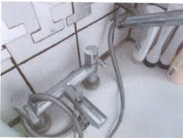
Bathroom - black spot mould around tiling/bath seal
