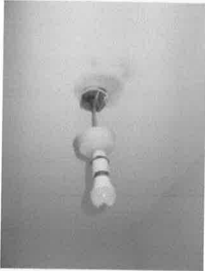
Defective ceiling mounted light fitting - lower ground floor hall (Observation)
