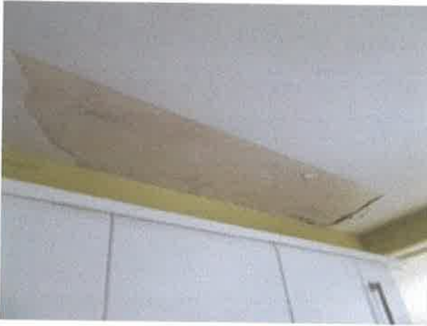
Kitchen - water damage to ceiling - incomplete repair
