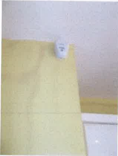
Kitchen - wall mounted CO alarm
