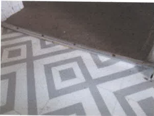
Kitchen - gap at threshold bar between kitchen and lower ground floor hall - trip hazard
