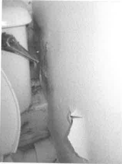
Bathroom - black spot mould to rear of cistern and paint peeling to wall
