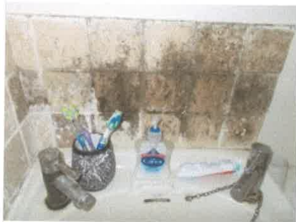
Bathroom - black spot mould around splash back tiles above wash hand basin
