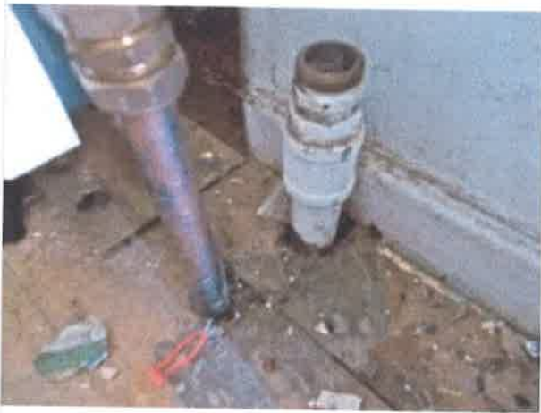
Cupboard off kitchen showing gas pipes/hole in floorboard
