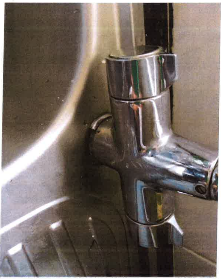
Damaged seal to kitchen tap
