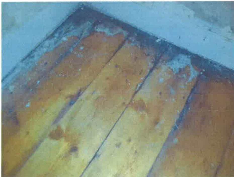
4 Staining and high moisture content to tongue and grooved flooring.
