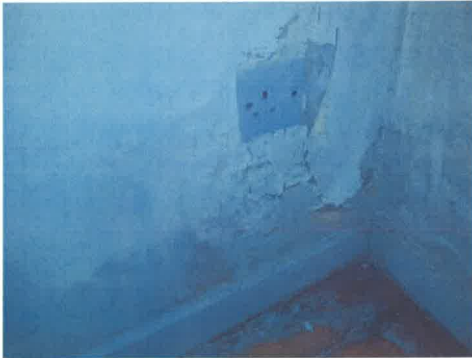
3 Failed decorative finishes due to saturation.
