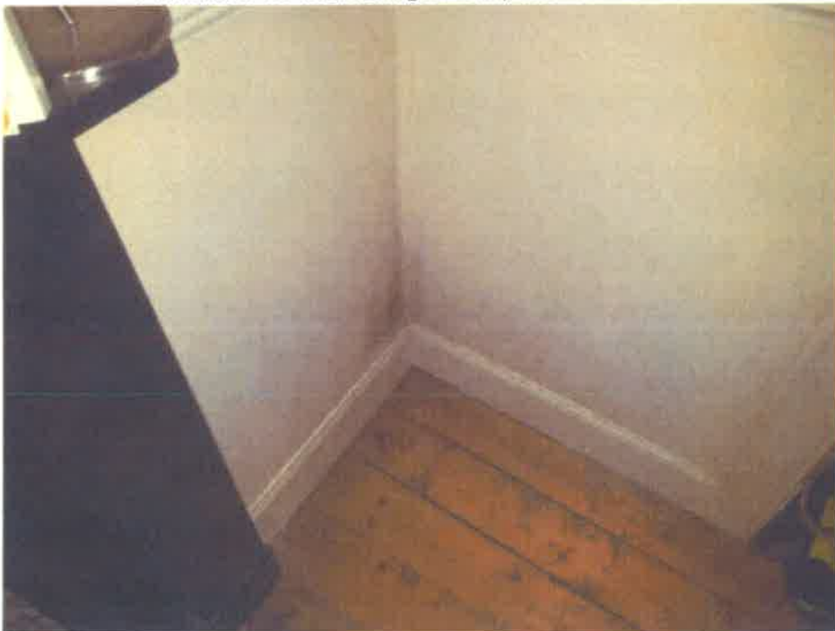
8 Mould growth to rear bedroom due to condensation. No high moisture readings.
