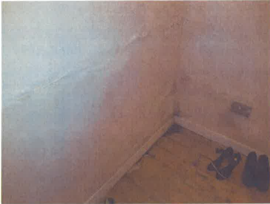
7 Evidence of low level staining and dampness within Boxroom.
