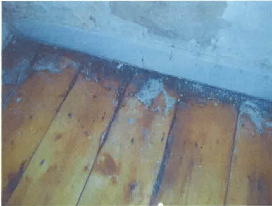
5 View of moisture transfer onto flooring from wall.
