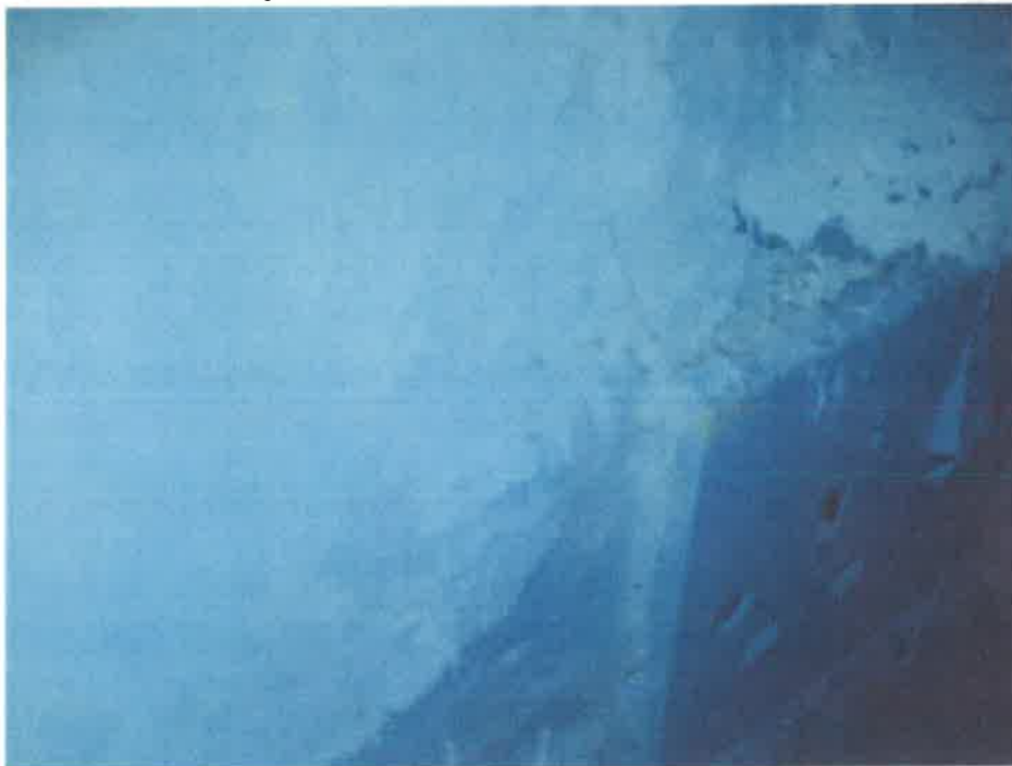
2 Close view of eruption of finishes due to water content.
