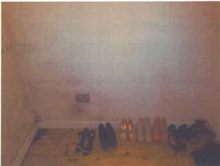
6 General view of low level staining within Boxroom.
