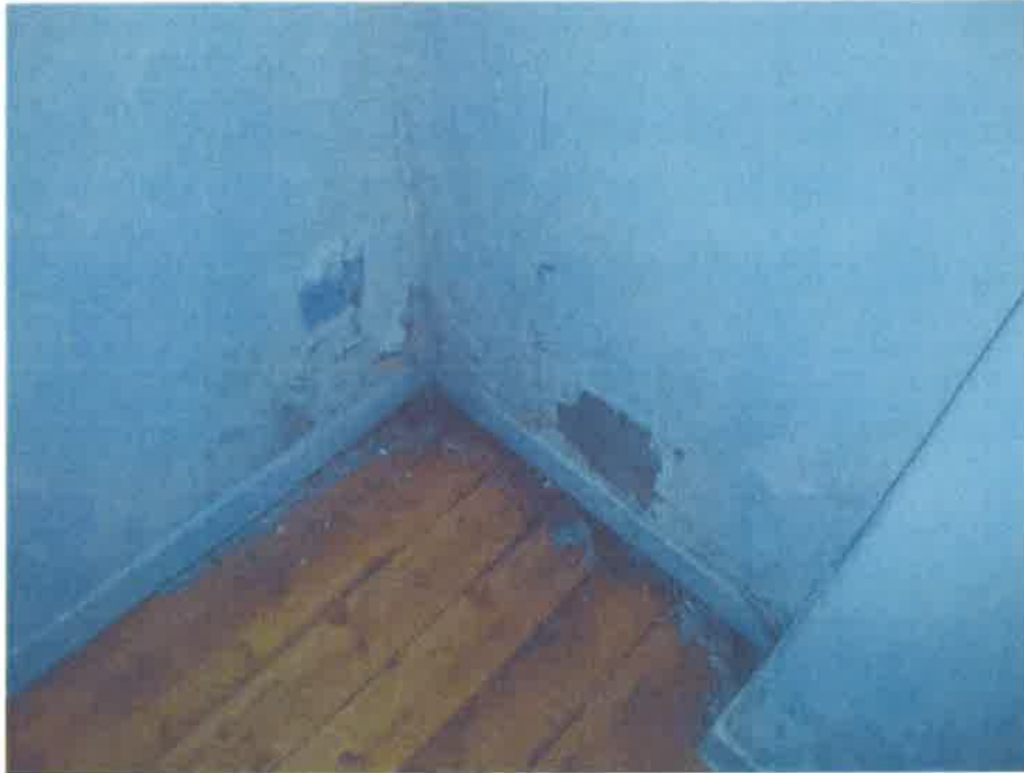
1 Rear corner of Living Room affected by low level dampness and high moisture readings.
