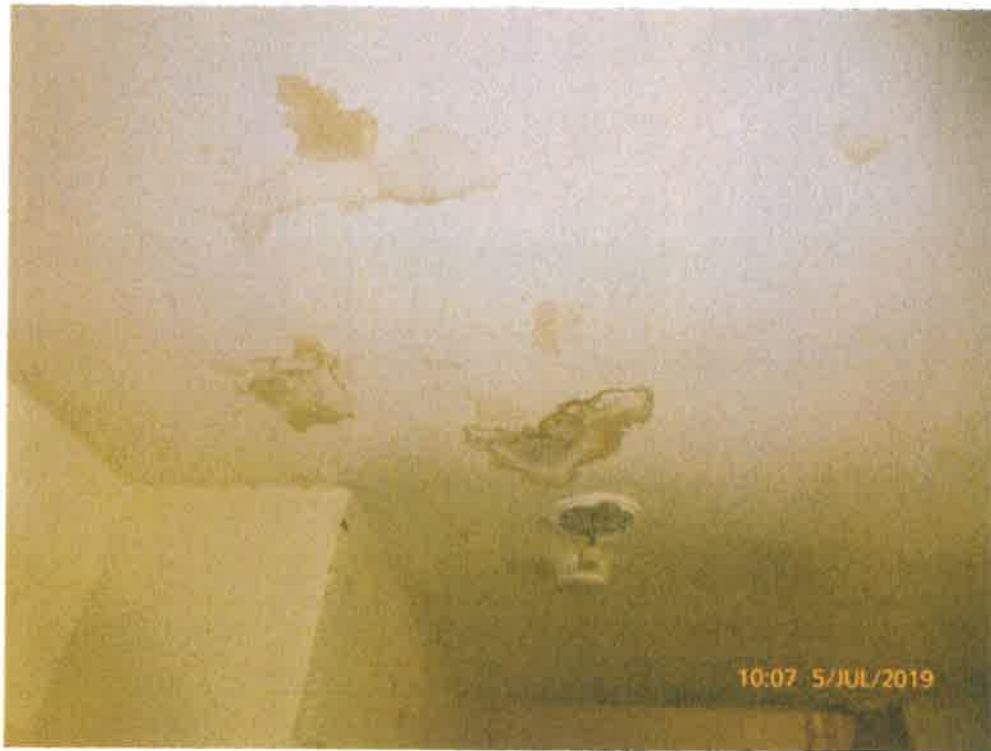
Various stains on the hall ceiling
