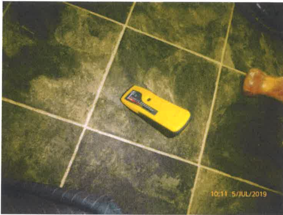
Dampness in the floor of the living-room
