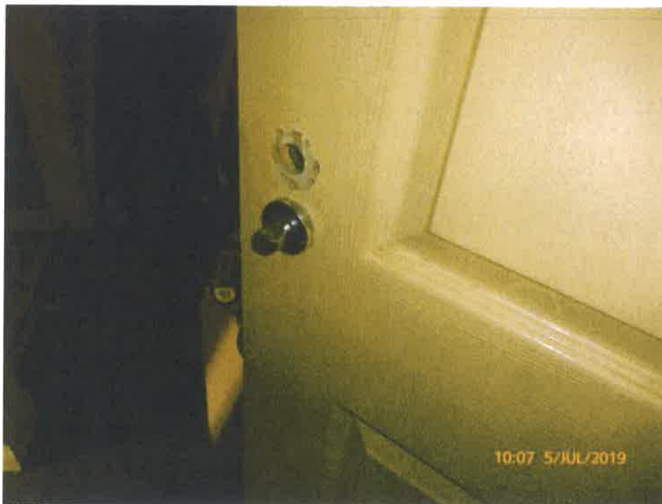
Door handle missing
