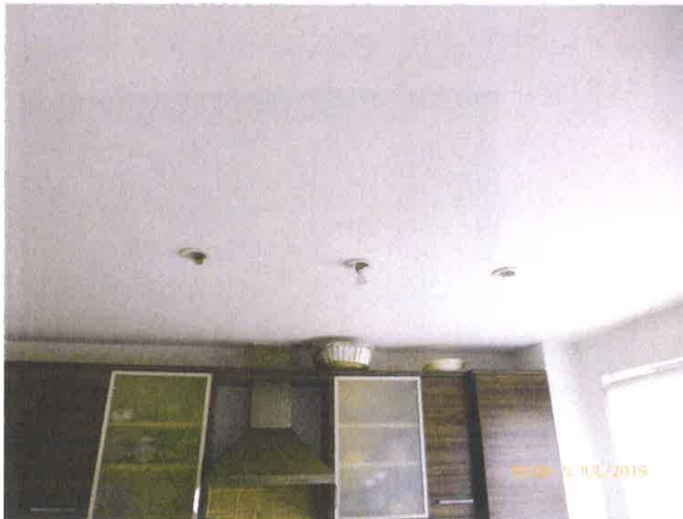
No heat detector in the kitchen
