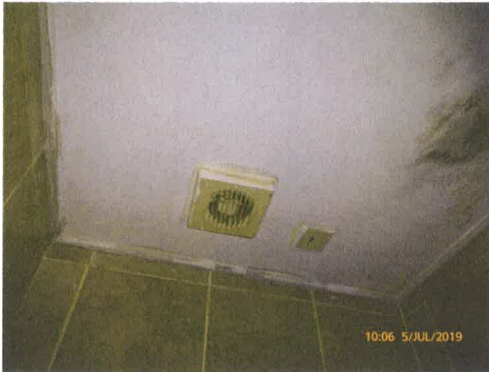
Fuse removed from extractor fan
