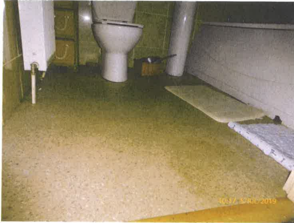
Water on the floor of the top floor bathroom
