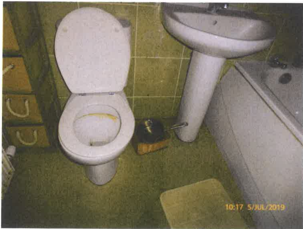
Pan collecting water from leak
