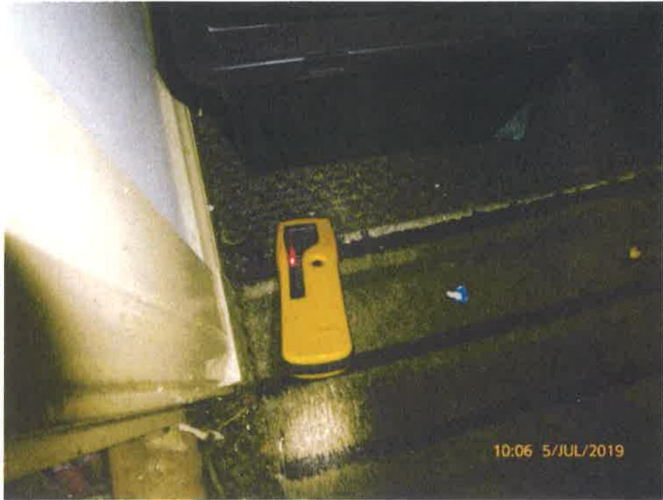
Dampness in the floor of the hall
