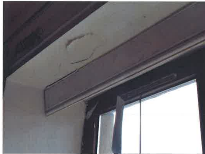
10. Staining and flaking paint above window in bedroom
