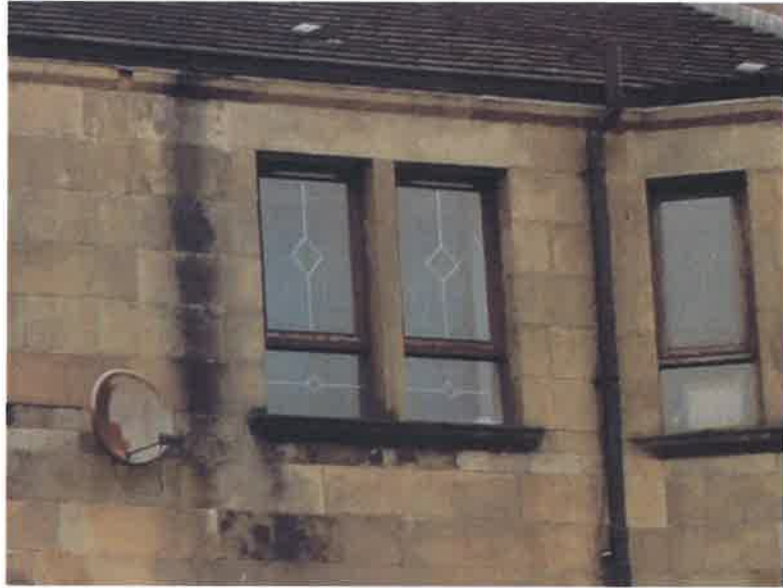
12 General wear and weathering at external window frame
