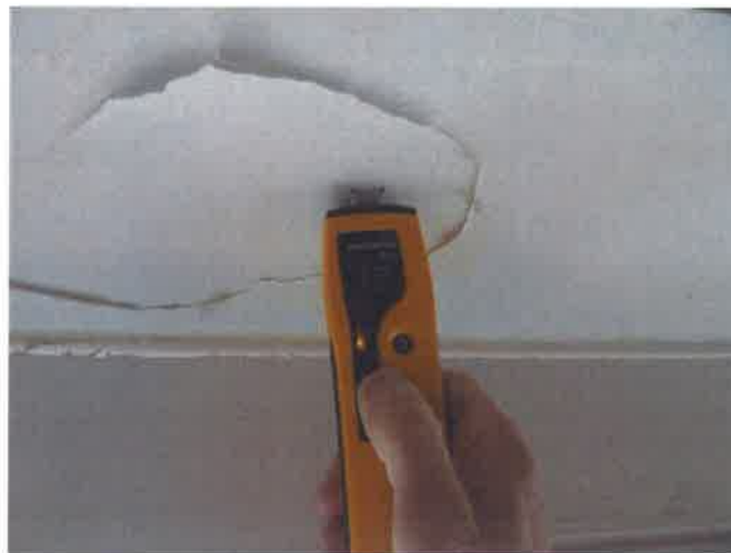
11. Moisture level of 18% above bedroom window
