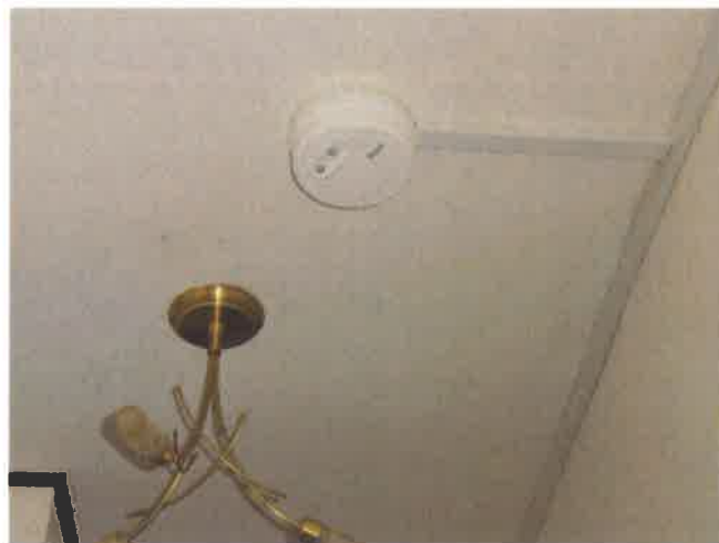
8. Mains wired smoke detector in hallway
