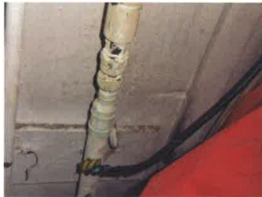
3. Exposed wiring at water tank
