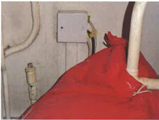
2. Wiring box at water tank
