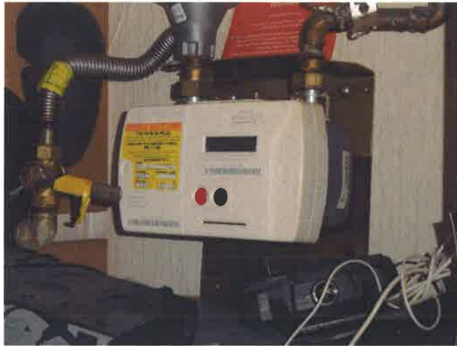
6. Non-operational gas tariff meter
