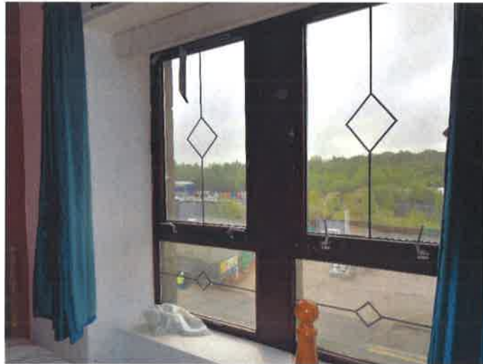
9. Bedroom windows with “PVC tape” as temporary draft / damp excluder
