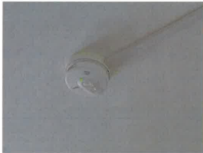
7. Mains wired smoke detector in living room
