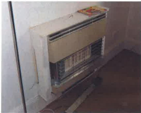
4. Baxi Bermuda "back boiler" (Gas fired)
