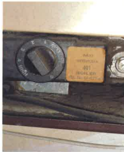
5. Baxi Bermuda "back boiler" (Gas fired)
