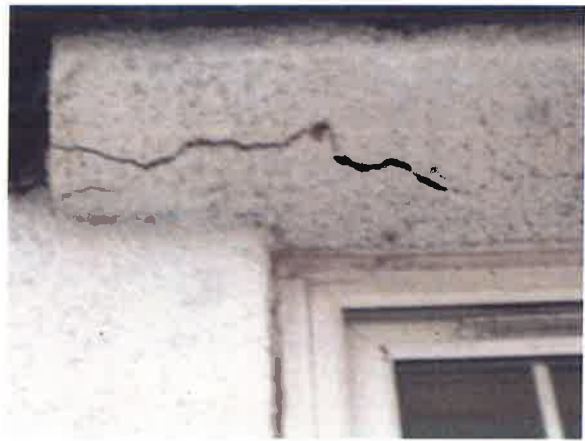
External - Front elevation - large crack to roughcast at eaves above front door/landing window
