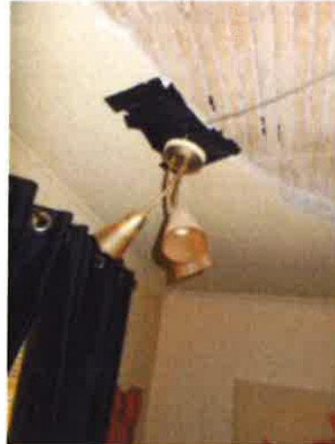
Living Room - ceiling mounted light fitting loose/taped by tenant adjacent to collapsed ceiling
