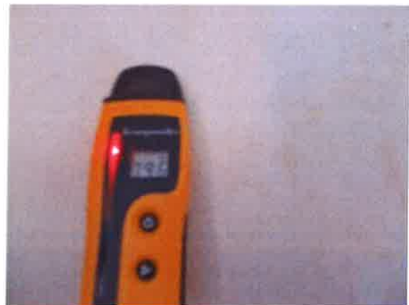
Rear Bedroom (2) high damp meter reading around damp patch on party wall to Bed (3), plaster crumbling under wallpaper
