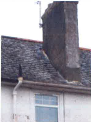
External - rear pitch of roof with chimney positioned above rear bedrooms (2) and (3)
