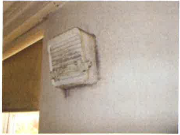
Kitchen - extractor fan - does not work
