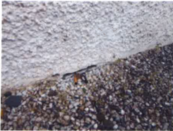
External - Gable Wall - underfloor vent below ground level
