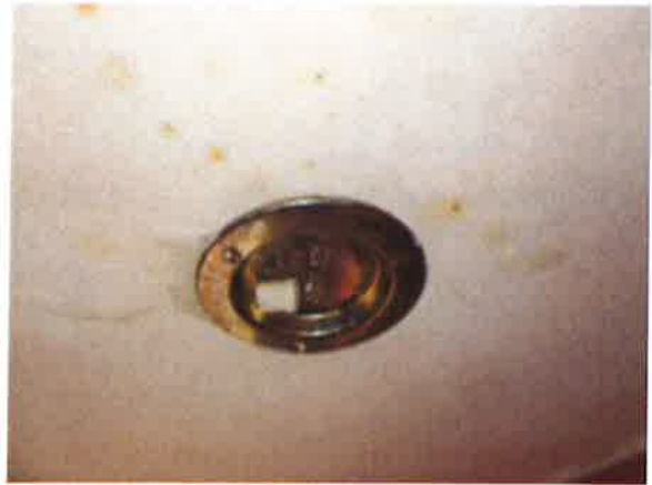
Bathroom - ceiling mounted light fitting defective/ damaged and not working
