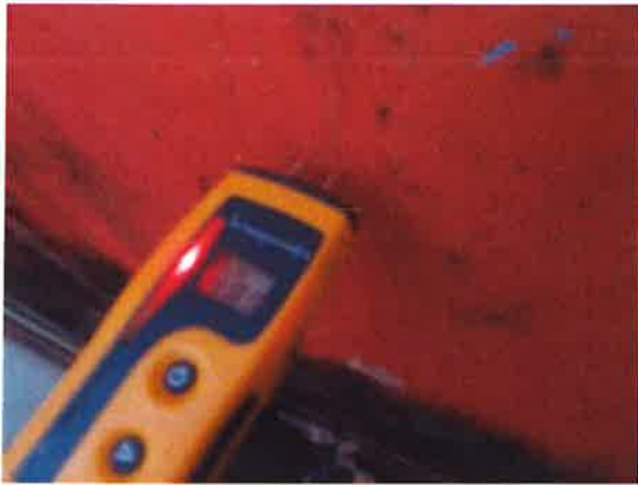
Bathroom - damp meter readings high to base of all walls - example shown on gable wall
