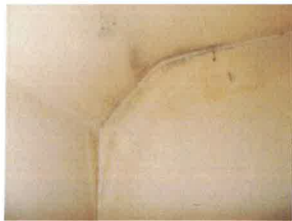
Front Bedroom (1) black spot mould in corner of ceiling at dormer window - left side
