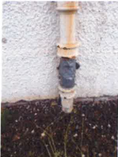
External - Front elevation - hole in cast iron downpipe covered with tape
