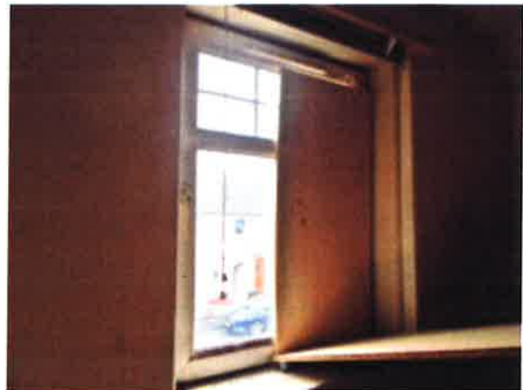
Front Bedroom (1) - window does not open properly, boards erected by tenant internally
