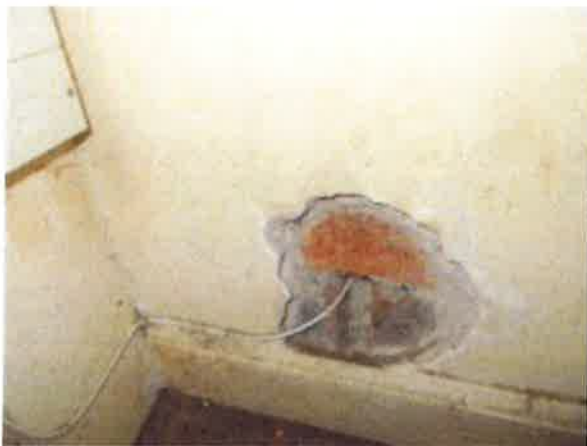
Hall - large hole in plaster at base of party wall to kitchen, brickwork exposed and wire protruding
