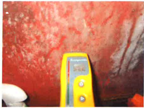
Bathroom - damp meter readings high to base of all walls - example shown on front elevation
