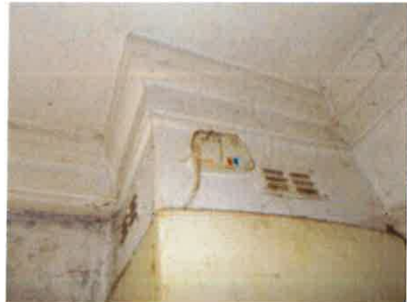
Kitchen - Wall mounted Carbon Monoxide alarm positioned just above the boiler
