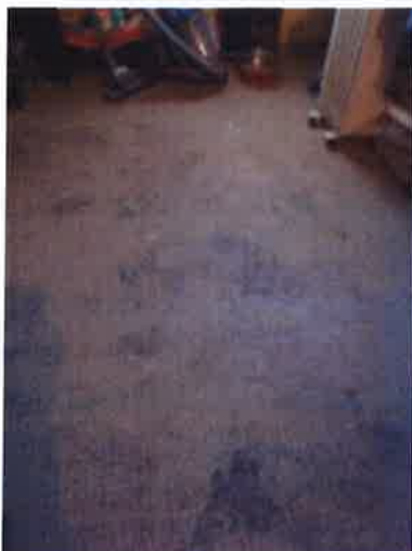
Living Room - Carpet worn and extensively stained
