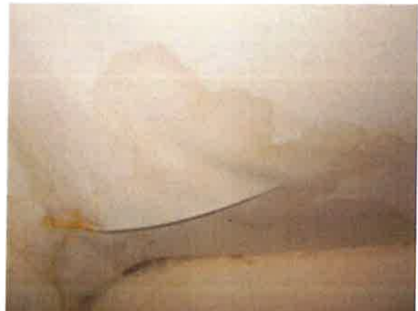
Rear Bedroom (2) - water staining to ceiling and wall towards rear elevation/party wall to Bed (3)
