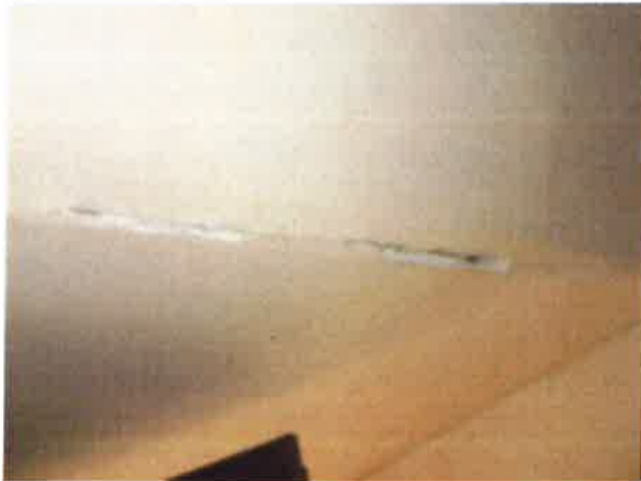
Hall - large crack in plaster ceiling above front door
