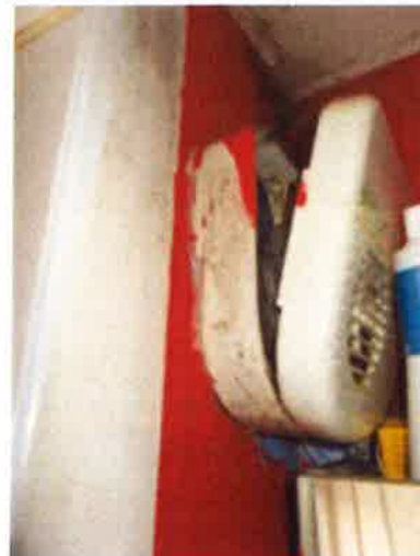
Bathroom - Extractor fan defective/damaged and not working
