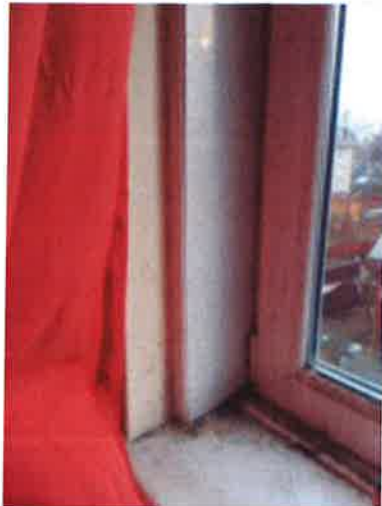
Rear Bedroom (2) - window - black spot mould around frame and sill
