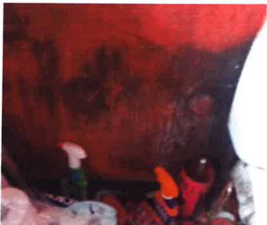
Bathroom - Extensive damp and condensation
