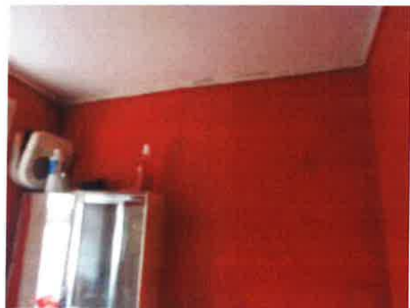
Bathroom - Extensive damp and condensation
