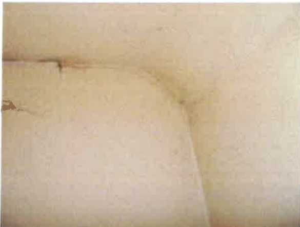
Front Bedroom (1) black spot mould in corner of ceiling at dormer window - right side
