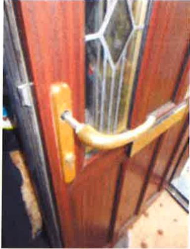
Front Door - external - handle loose, not fixed properly
