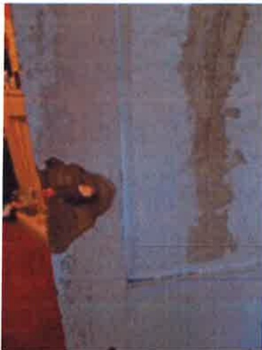
Living Room - door damaged/no handle
