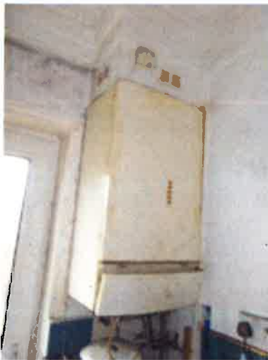
Kitchen - Boiler wall mounted on rear external wall
