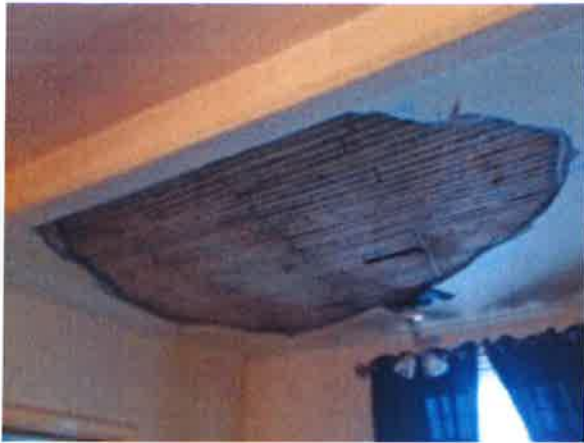
Living Room - large section of ceiling collapsed - plaster missing and lath exposed
