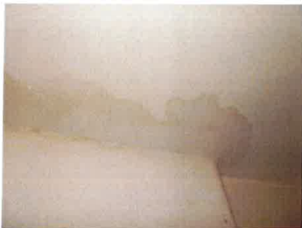
Rear Bedroom (2) - water staining to ceiling at party wall
