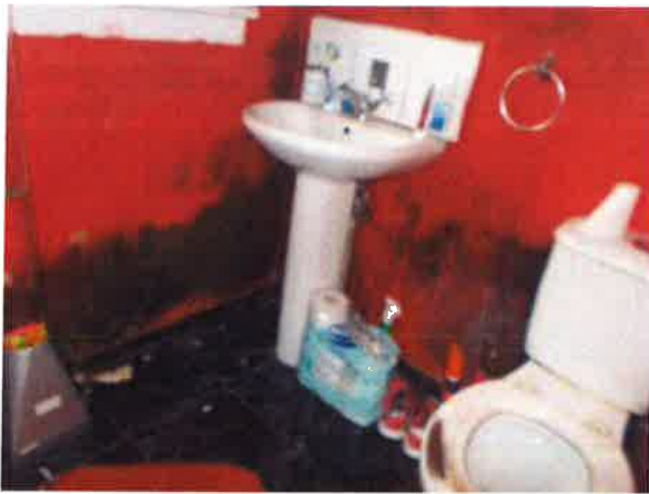
Bathroom - Extensive damp and condensation
