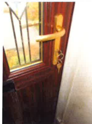
Hall - Front door handle defective, key will not turn in lock
