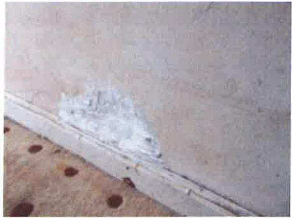
Hall - hole in plaster at base of party wall to LR, part filled with mastic by tenant
