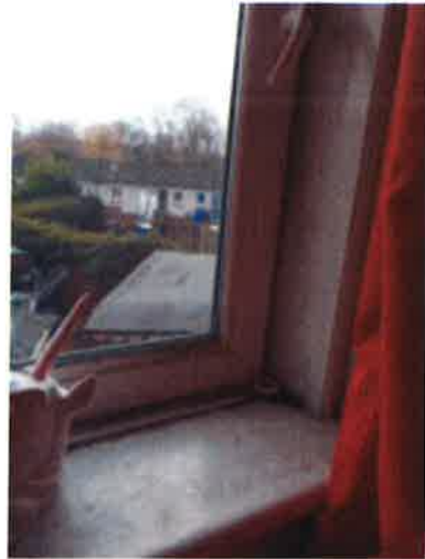
Rear Bedroom (2) - window - black spot mould around frame and sill
