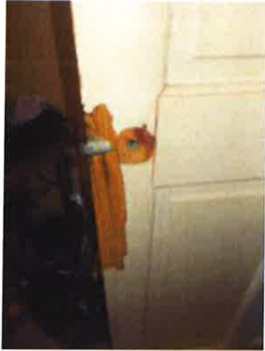
Front Bedroom (1) - door damaged and handle missing
