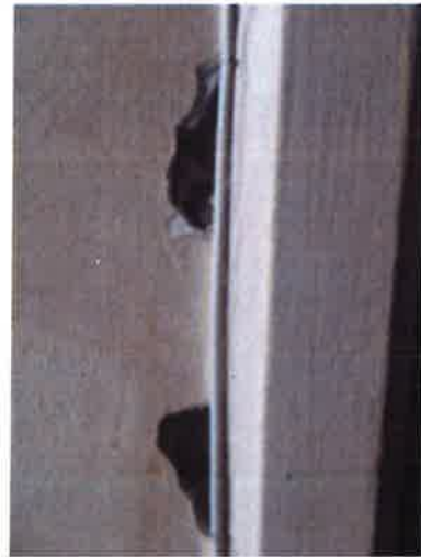
Hall - holes in plaster to left side of living room door
