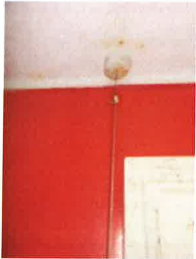
Bathroom - pull cord damaged
