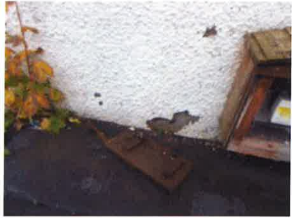
External - Gable Wall - patches of roughcast spalling
