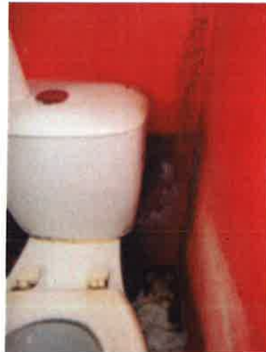
Bathroom - Extensive damp and condensation
