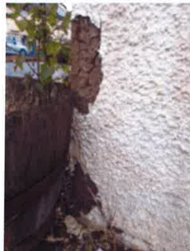
External - Gable Wall - patches of roughcast spalling
