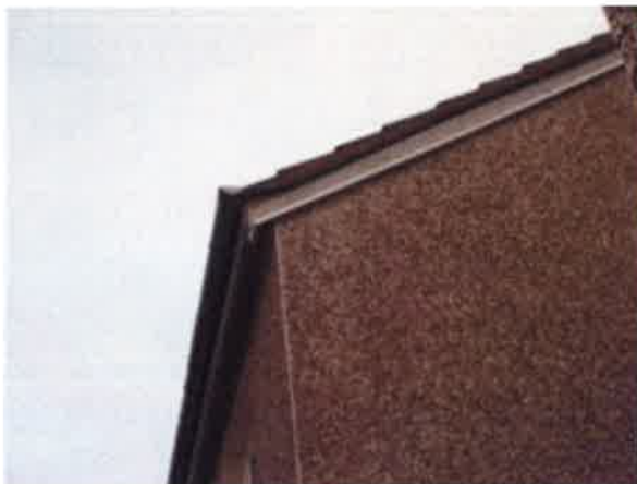
Verge on gable - mortar missing towards corner of front elevation
