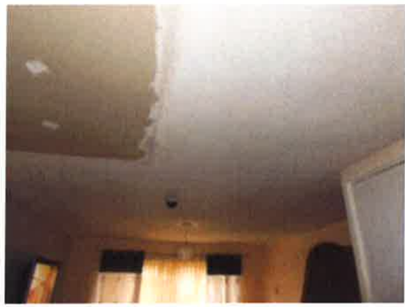
Living Room - Repair to ceiling incomplete/new section of plasterboard exposed/no decoration
