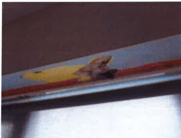
Kitchen - plaster damaged/hole above window
