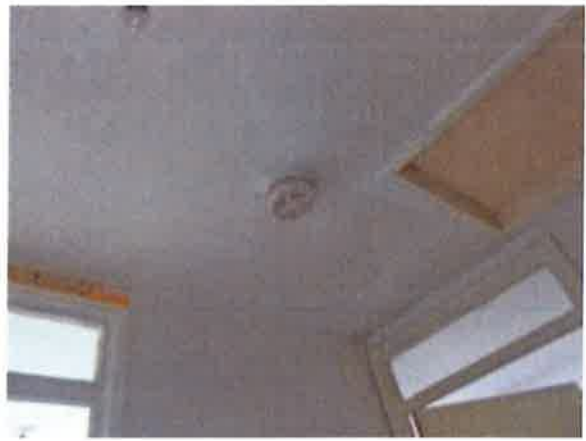
Landing - Ceiling mounted Smoke Alarm
