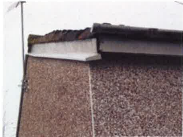
Verge on gable towards rear elevation -mortar missing and gaps/possible rot to fascia boards
