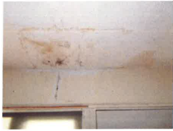
Kitchen - Ceiling water stained and plaster damaged
