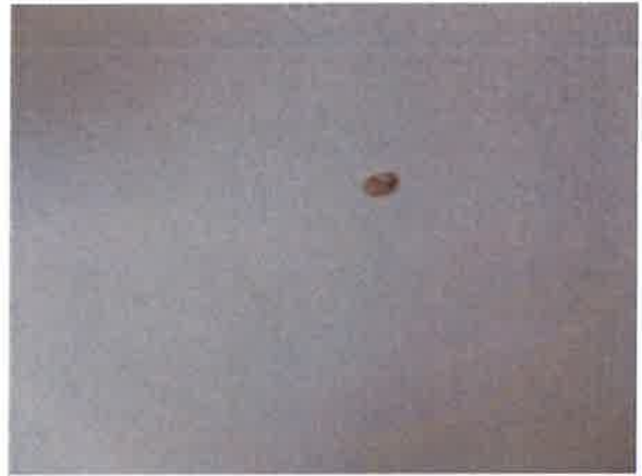
Rear Bedroom (1) Hole in ceiling
