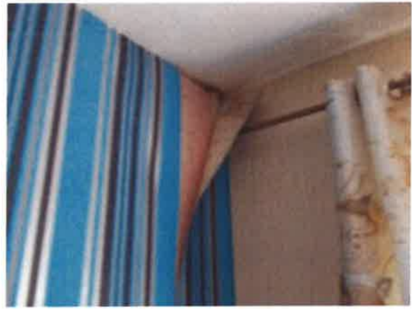
Front Bedroom (2) - Wallpaper peeling and black spot mould to front corner at gable wall
