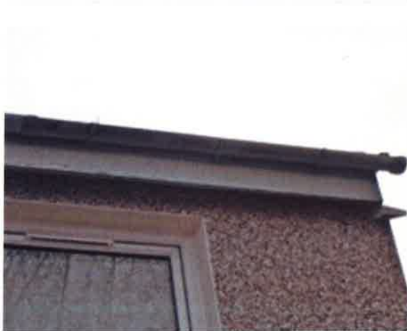
Front Elevation - gutter leaking and vegetation growth
