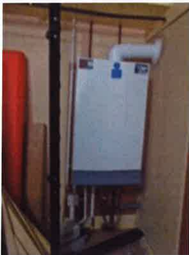
Front Bedroom (2) Boiler housed in cupboard
