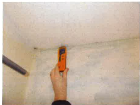
Rear Bedroom (1) Damp meter reading amber - gable wall at ceiling
