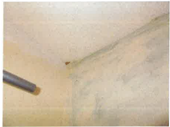
Rear Bedroom (1) Black spot mould rear corner at gable wall
