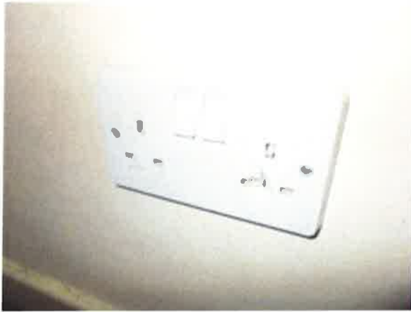
Rear Bedroom (1) Damaged socket cover
