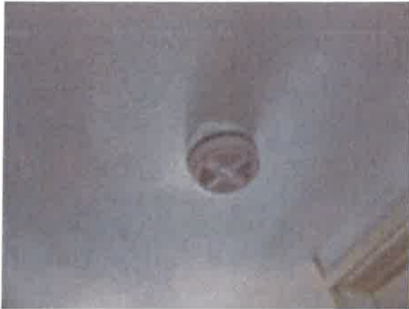
Hall - Ceiling mounted Smoke Alarm
