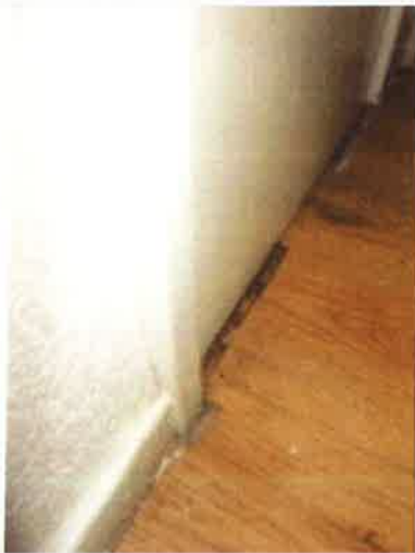
Hall - Gaps in laminate floor covering around skirting boards
