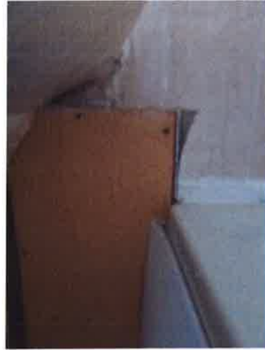
Bathroom - poor quality boxing of pipes/bath seal defective
