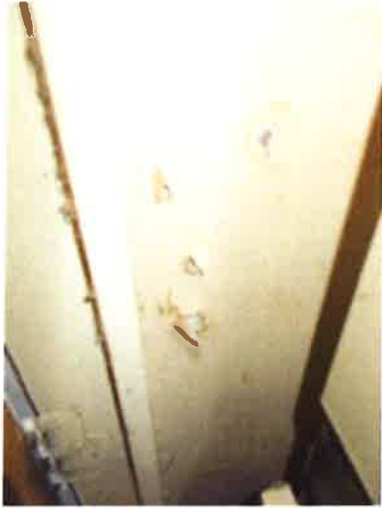
Living Room - some damage to wall lining in cupboard housing obsolete warm air heating system
