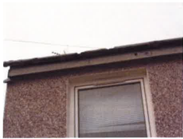
Rear Elevation - gutter broken in several places and vegetation growth
