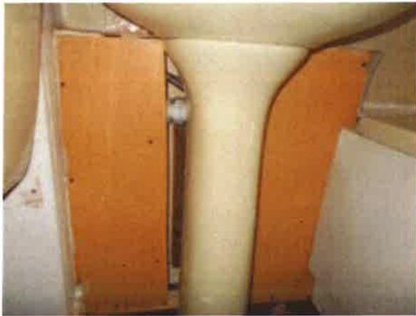
Bathroom - poor quality boxing of pipes under wash hand basin
