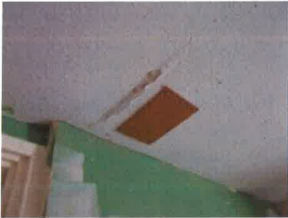
Rear Bedroom (1) Hole in ceiling covered by tenant
