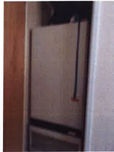
Living Room - obsolete warm air heating system
