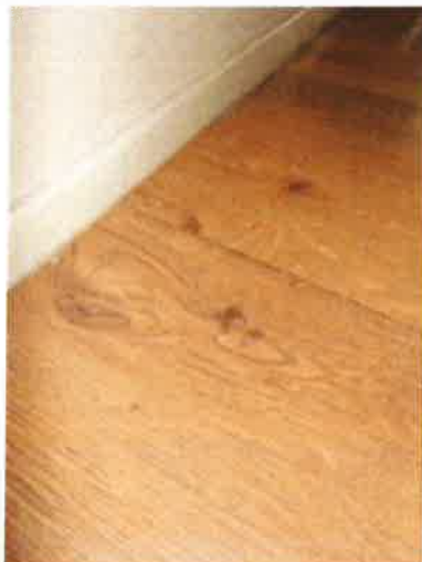
Hall - Uneven laminate floor
