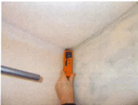
Rear Bedroom (1) Damp meter reading amber - rear corner at gable wall
