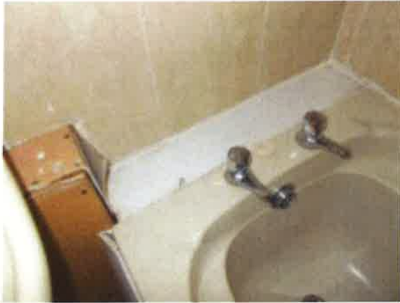
Bathroom - poor quality boxing of pipes/bath seal defective
