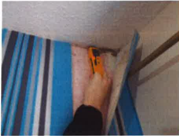
Front Bedroom (2) - Damp meter reading - amber to front corner at gable wall
