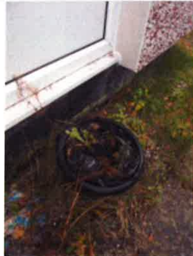
Front Elevation - gutter leaking, dripping into planter
