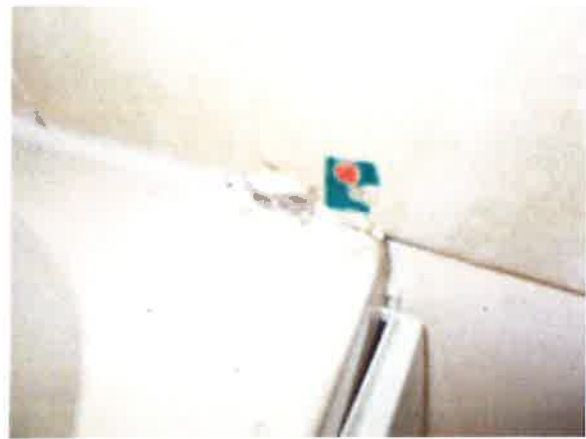
Bath panel poorly fitted, loose and gaps. Bath seal defective
