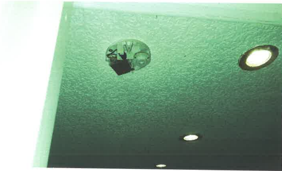
5 The defective smoke detector in the entrance hall
