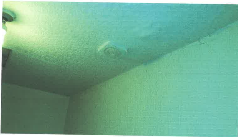
6 The blocked off extract ventilation fan in the bathroom
