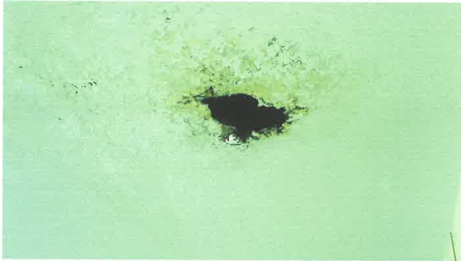
1 The hole in the lounge/kitchen ceiling due to water penetration
