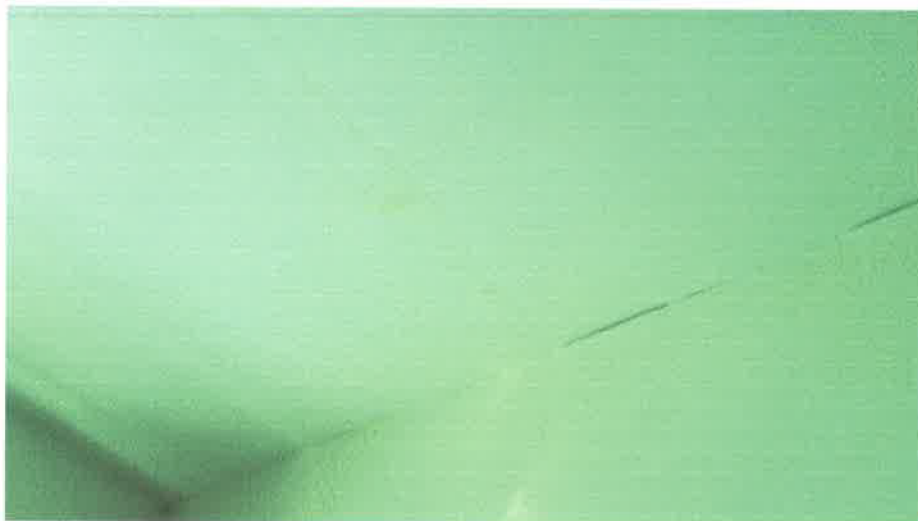
2 The evidence of water penetration in the bedroom ceiling
