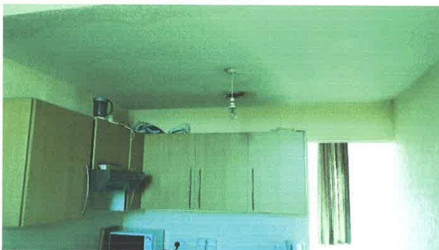
3 The absence of heat detector in the lounge/kitchen
