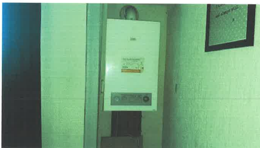
4 The absence of a carbon monoxide detector in the vicinity of the gas boiler
