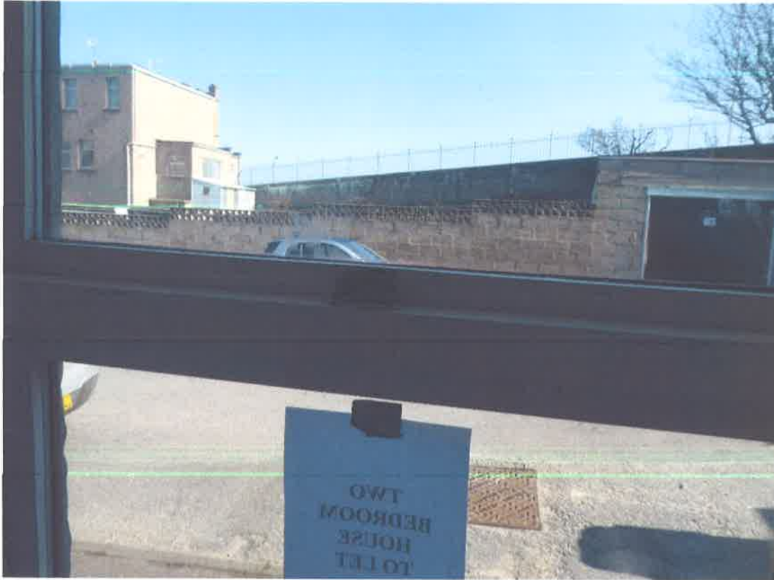
Ground floor left hand window – broken catch
