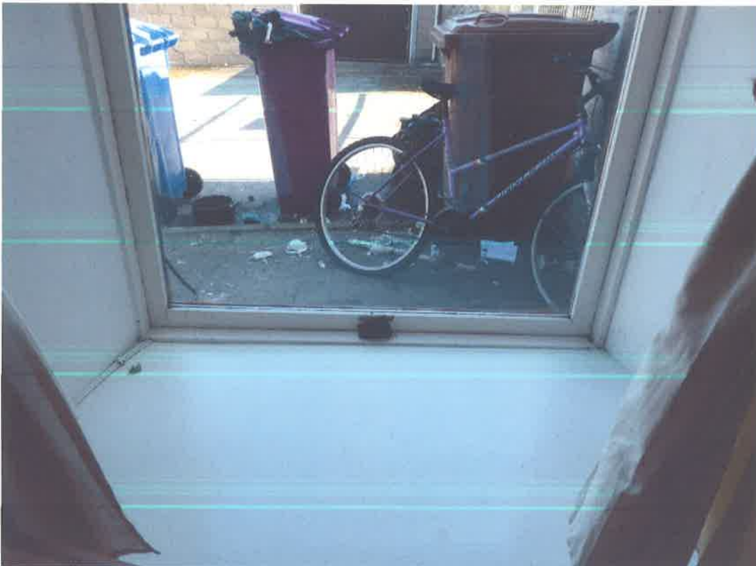
Ground floor right hand window – broken catch
