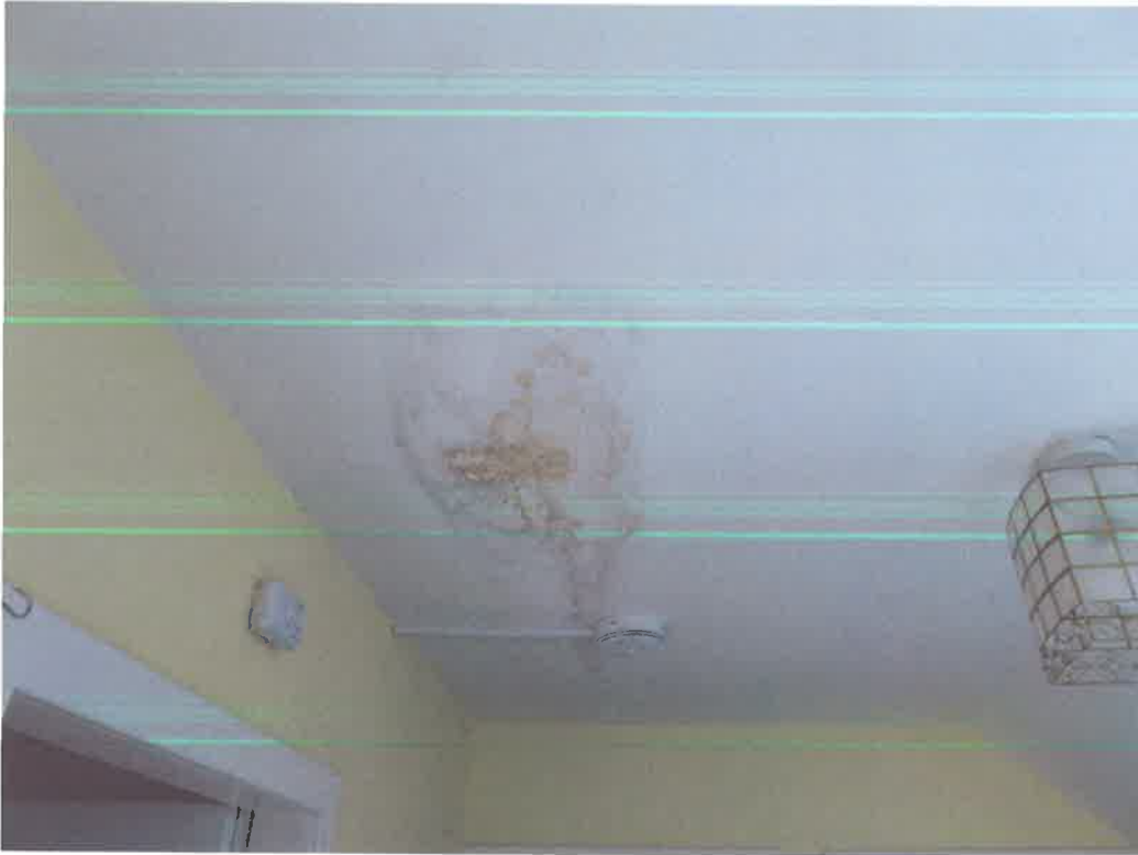
Ceiling on 1 st floor landing showing leak from flat roof above
