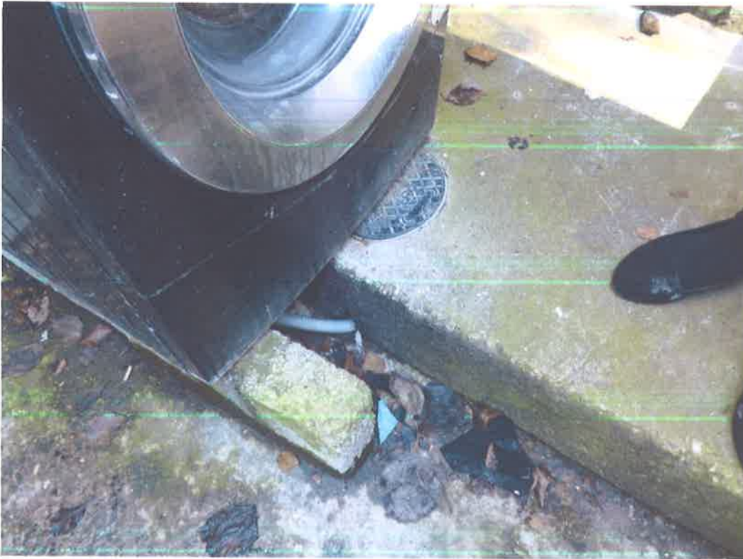
Method of drainage employed by former tenants for washing machine (outside) – to be removed and drain sealed to prevent smells and potential leakage of foul water.
