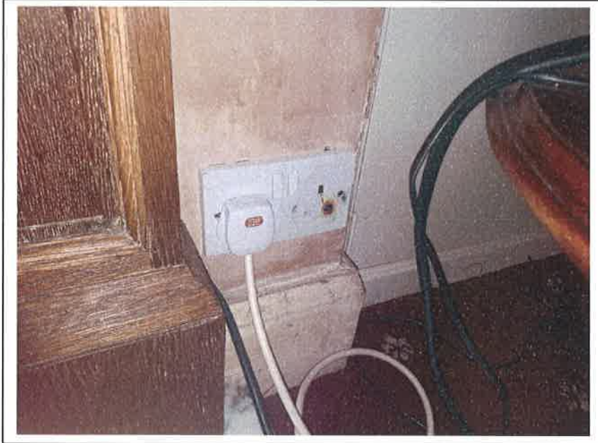
Damaged socket in living room
