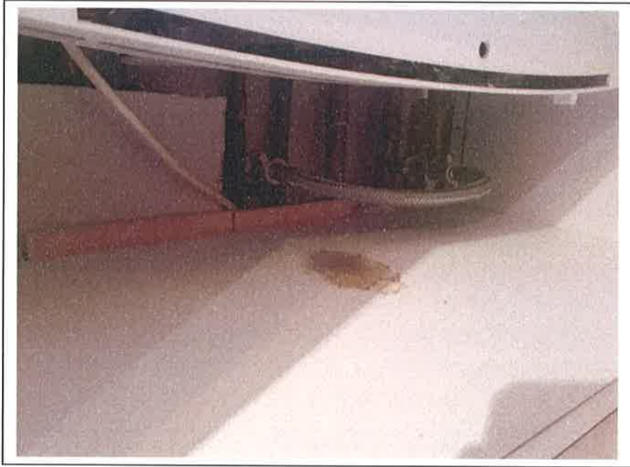
Water staining below boiler
