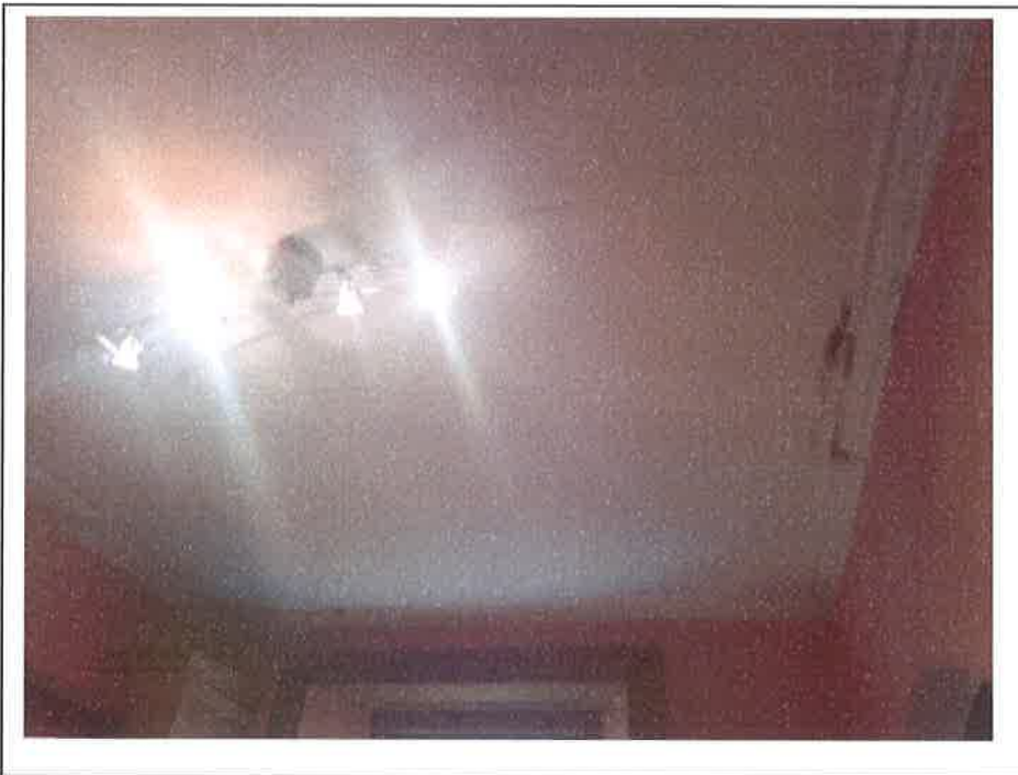
Damp staining - kitchen ceiling
