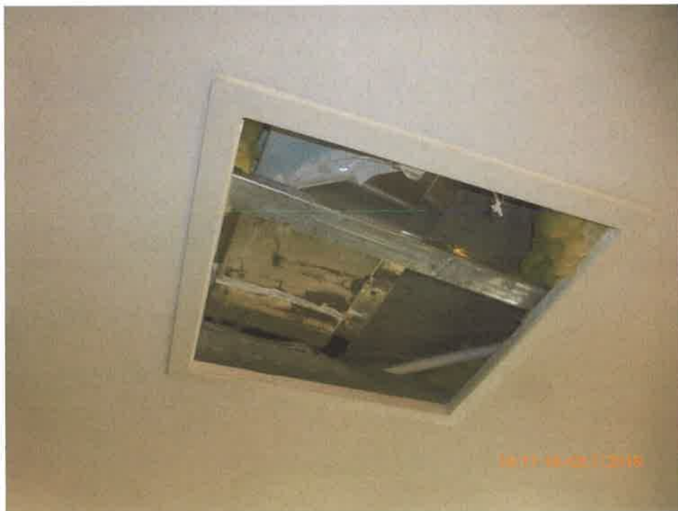
Detail showing the faulty joint in the drain (with white temporary seal)
