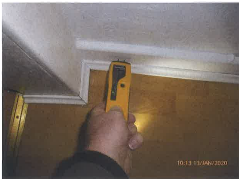
Damp meter reading
