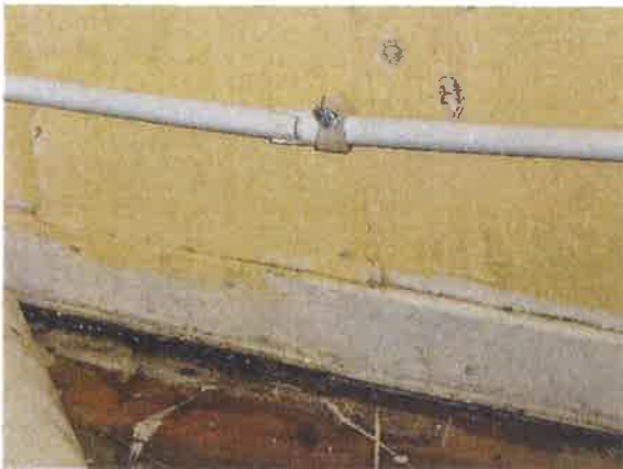
Sagging pipe 5 Nov 2019
