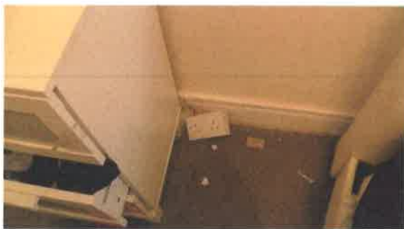
Photo 4 – Damaged socket in bedroom
