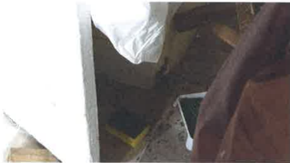
Photo 2 – Rodent hole + missing skirting
