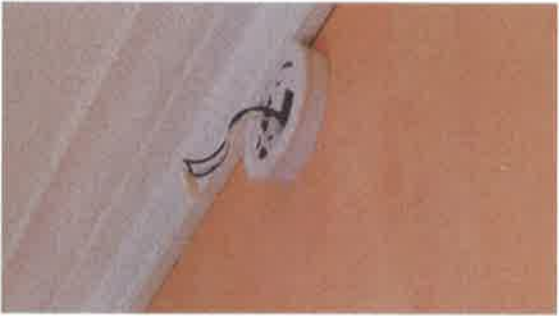
Photo 10 – Defunct smoke alarm in hall
