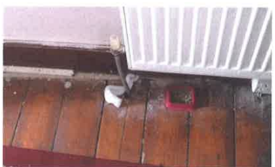
Photo 7 - Rodent access in living room
