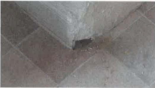
Photo 6 – Rodent hole/missing skirt.
