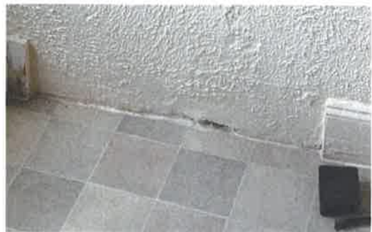
Photo 3 – Rodent hole + missing skirting
