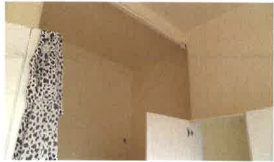
Photo 9 – Example of poor decorating
