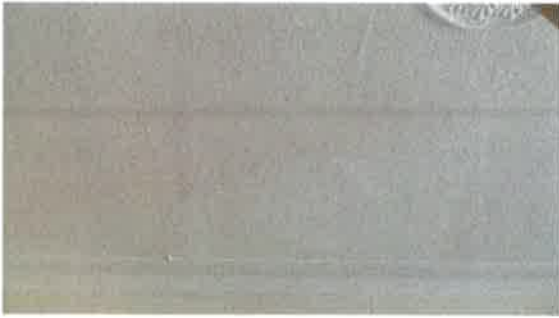
Photo 8 – Papered-over hole in L/R ceiling
