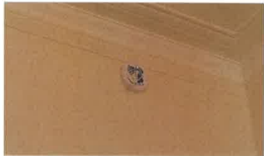
Photo 11 – Defunct smoke alarm in L/R
