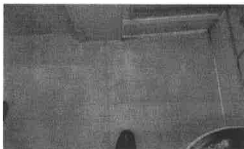
Photo 7 – Slight dampness in floor
