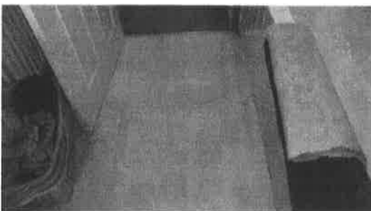
Photo 6 – Floor section at door now dry
