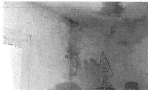
Photo 3 – Noted at inspection 03/06/19
