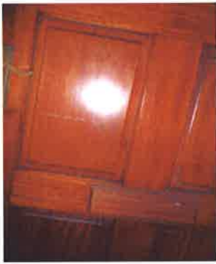
8. Back door showing splits in panels
