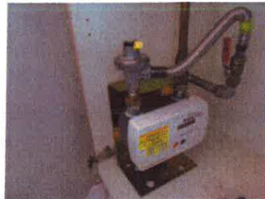
Kitchen - new gas meter and bracket
