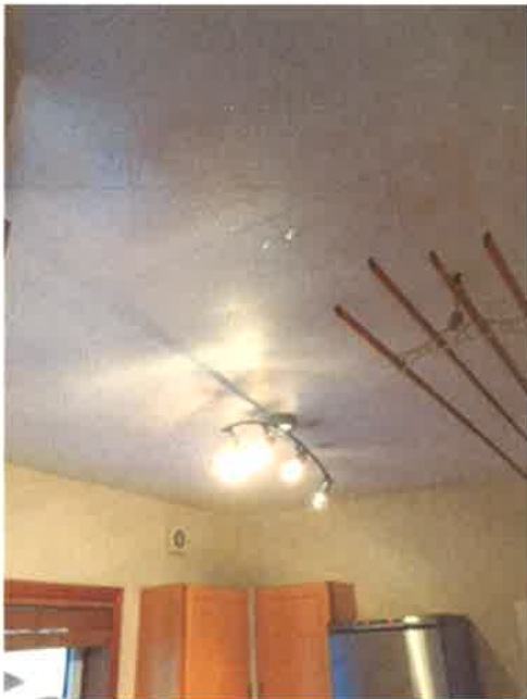
Kitchen ceiling - no smoke detector
