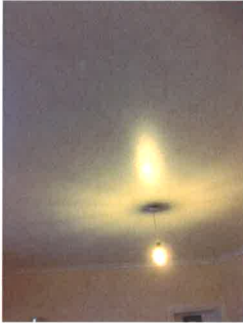
Living Room ceiling - no smoke detector
