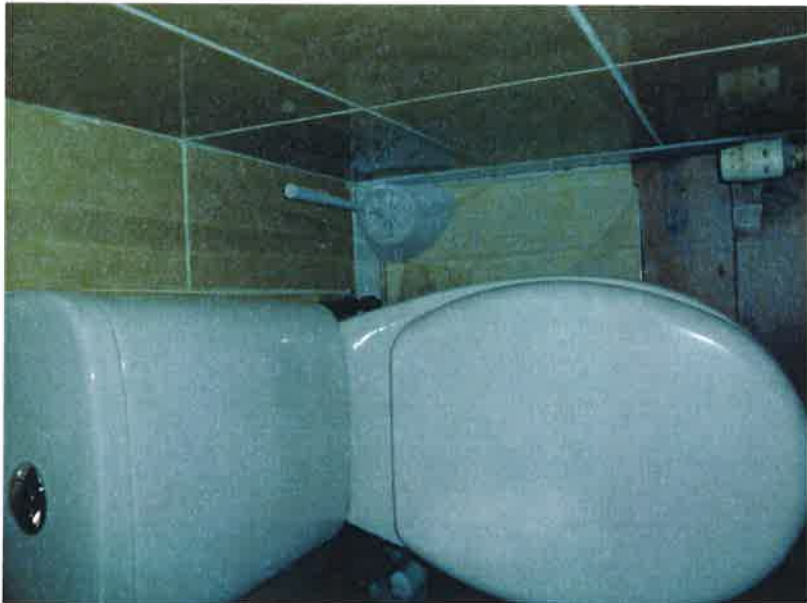
Leak at WC – December 2016
