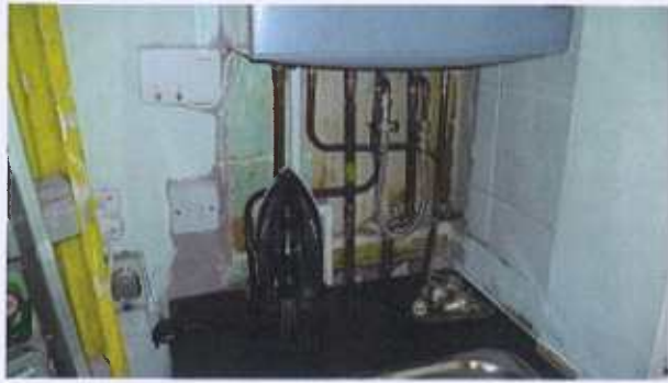
(Ph16) Kitchen – Boiler + pipework
