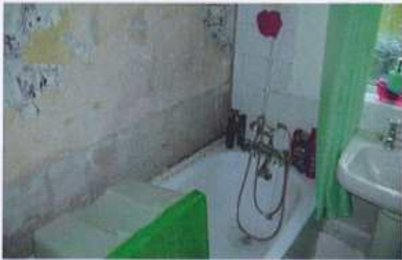
(Ph5) B/R – Missing tiles/bath seal
