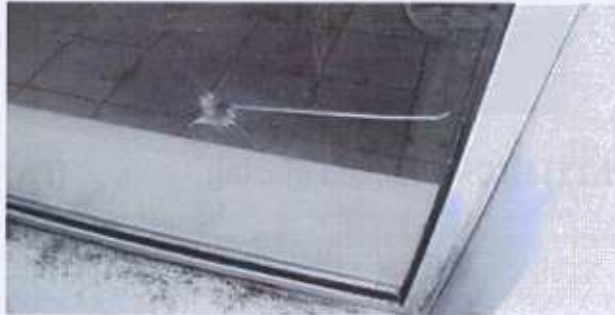
(Ph18) Bed 1 – Broken outer glass pane
