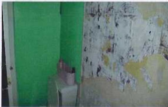
(Ph6) B/R – Missing tiles
