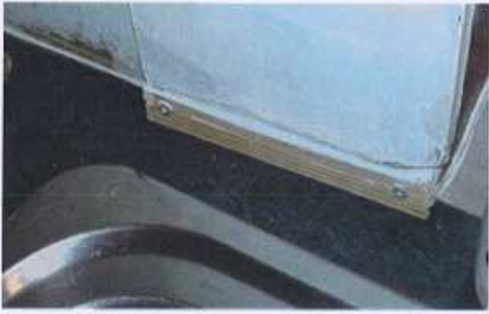
(Ph15) Kitchen – Patch behind sink
