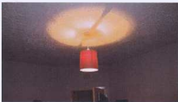
(Ph20) Bed 1 – Operational ceiling light
