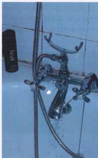
(Ph8) B/R - Cascading water from S/H
