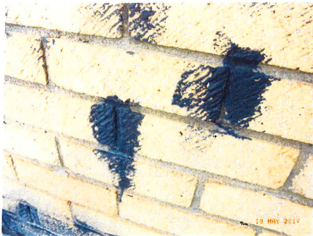
Joints in brickwork below Lounge window
