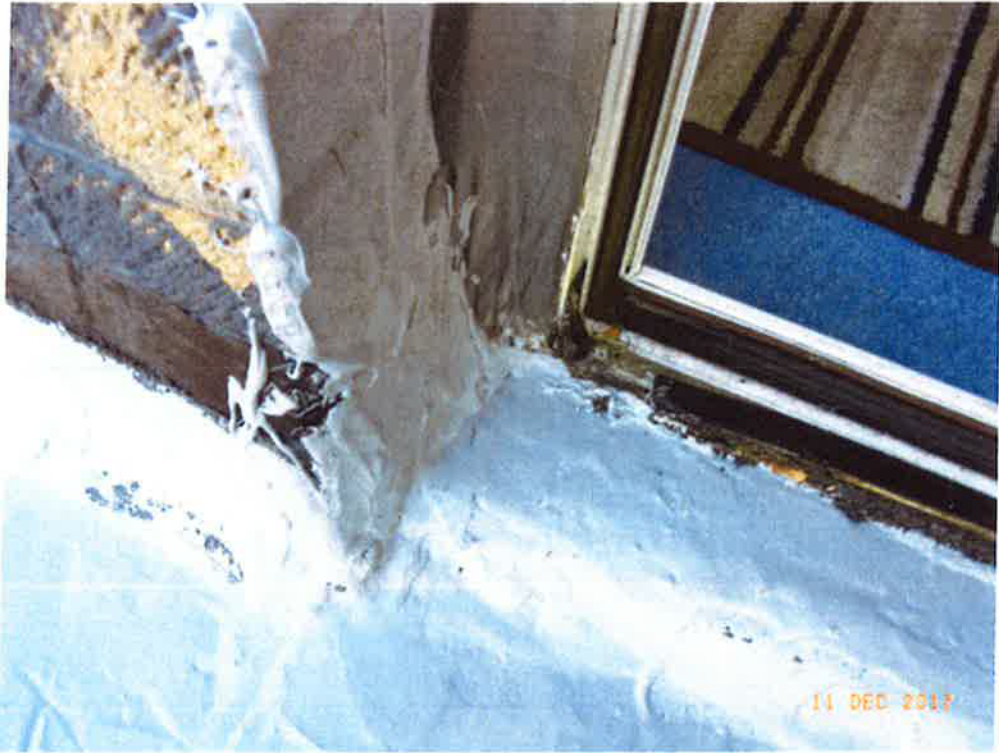
Lounge door – flashing at threshold
