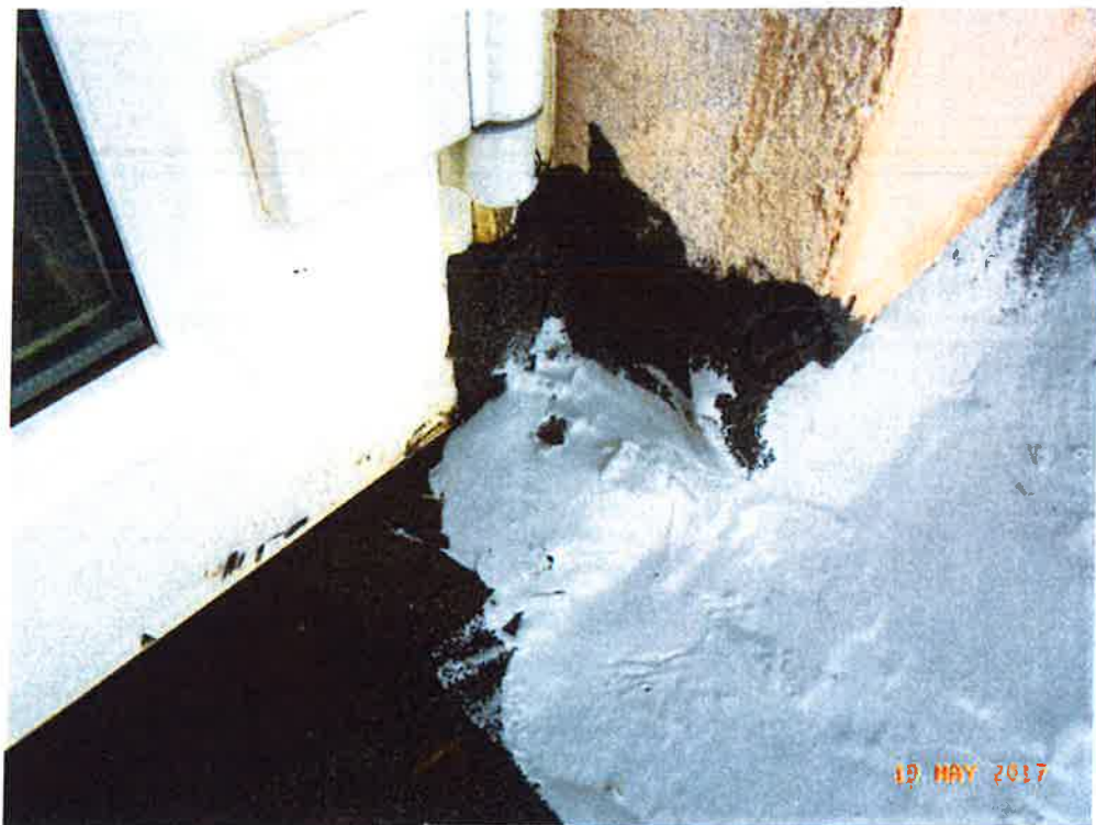
Lounge door – flashing at threshold
