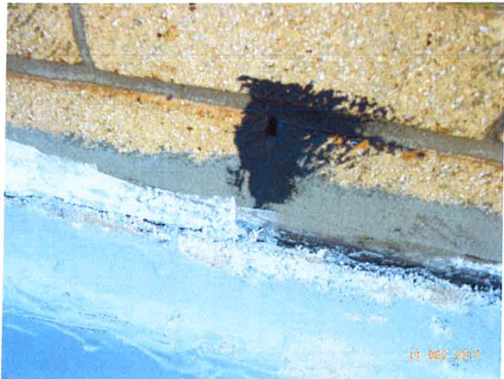
Joints in brickwork below Lounge window
