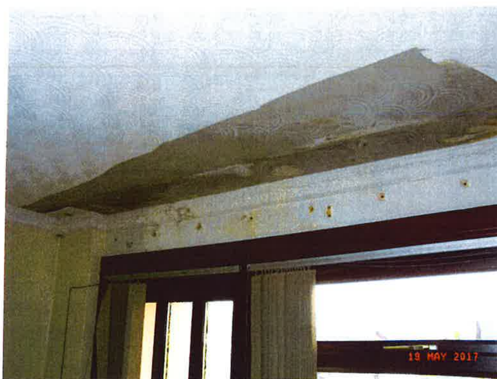
Ceiling of flat below
