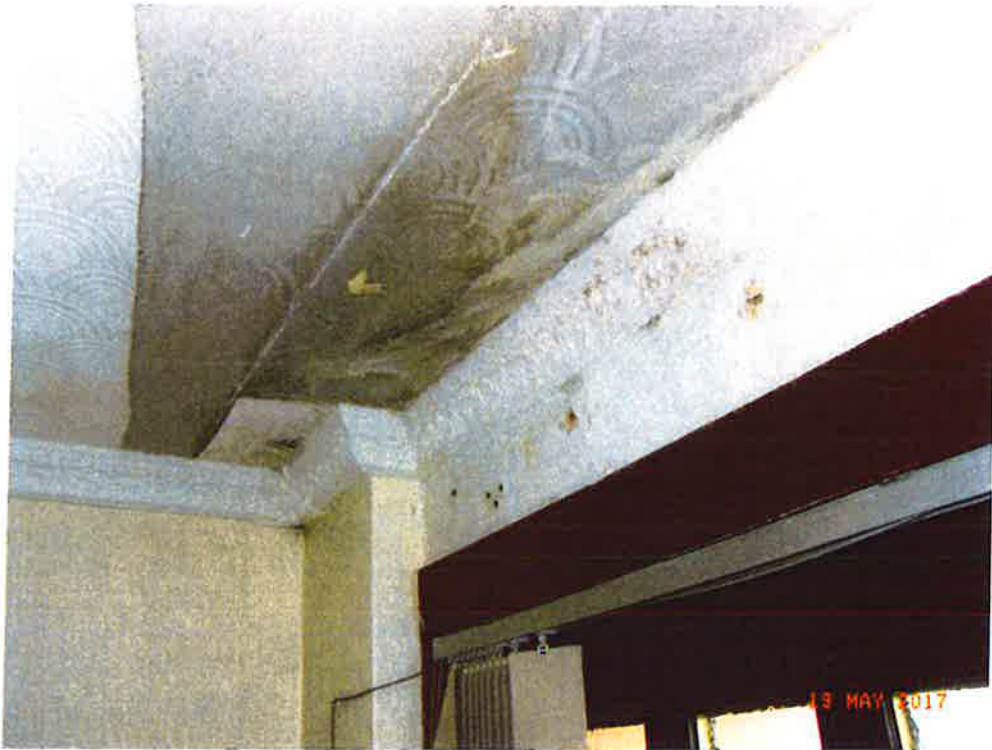
Ceiling of flat below (2)
