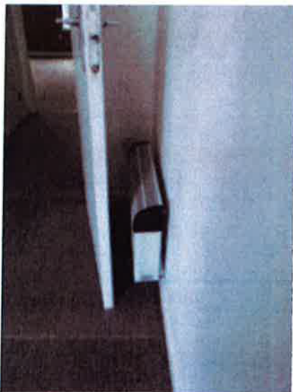
Dining Room - electric wall mounted heater
