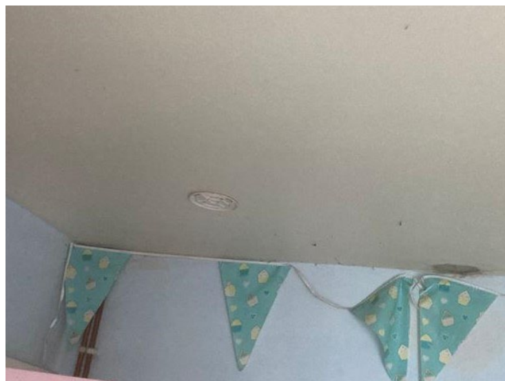
(b) Kitchen ceiling with no visible functioning heat detector 28 June 2022
