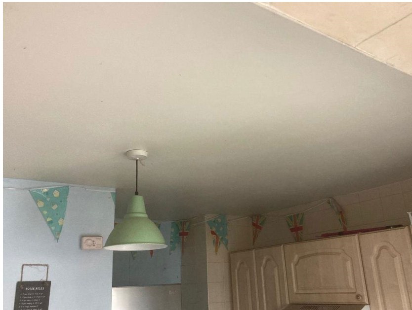
(c) Kitchen ceiling with no visible functioning heat detector 28 June 2022
