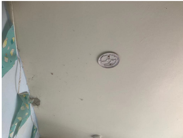
(a) Kitchen ceiling with no functioning heat detector 21 April 2022
