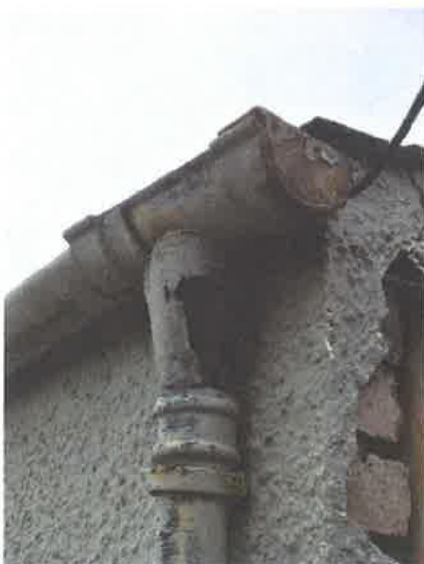
Defective rain water goods and rendering 1 st October 2019
