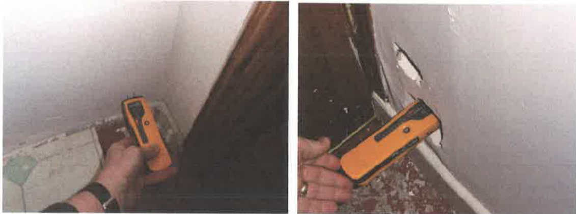
Damp either side of front door with wall plaster to the right of the base of the entrance door collapsing due to saturation 28 th January 2020
