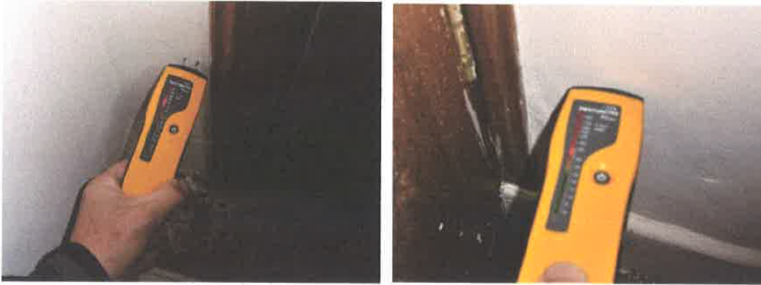
Damp either side of front door – 1 st October 2019
