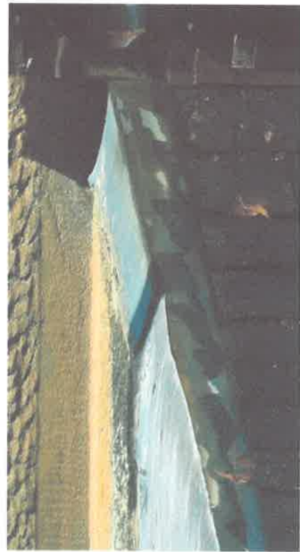
Photo 9 Flashing issue on rear dormer
