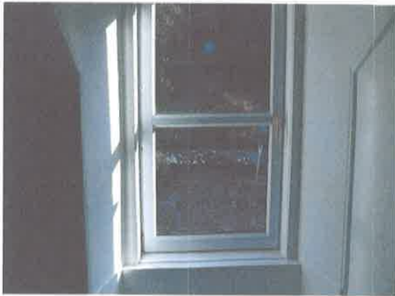
Photo 4 Dampness around window R/Bed
