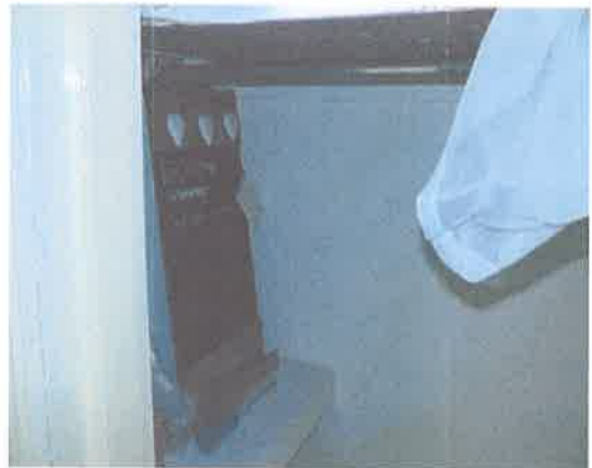
Photo 5 Saturated wall R/Bed cupboard
