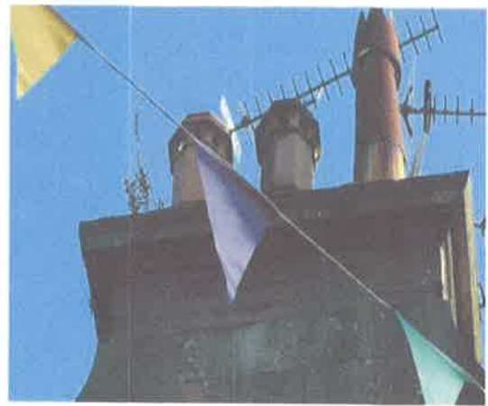
Photo 11 Vegetation on chimney cope
