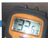
2d) Higher readings closer to skirting board – 33 in right hand corner, dropping to 29 in left hand corner.
