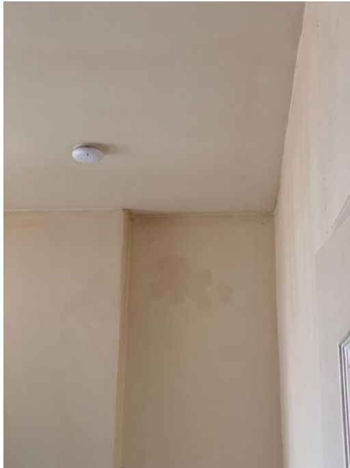
Photograph 2: Living room – smoke detector
