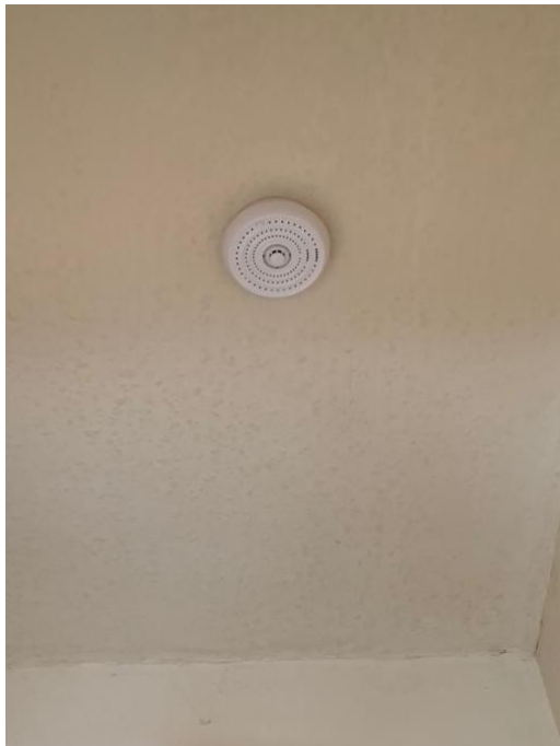
Photograph 3: Kitchen - heat detector
