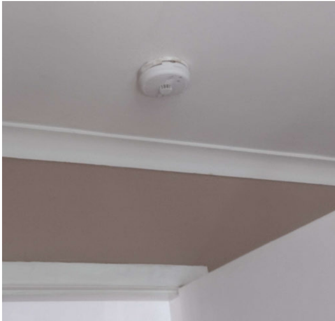
Heat detector in kitchen
