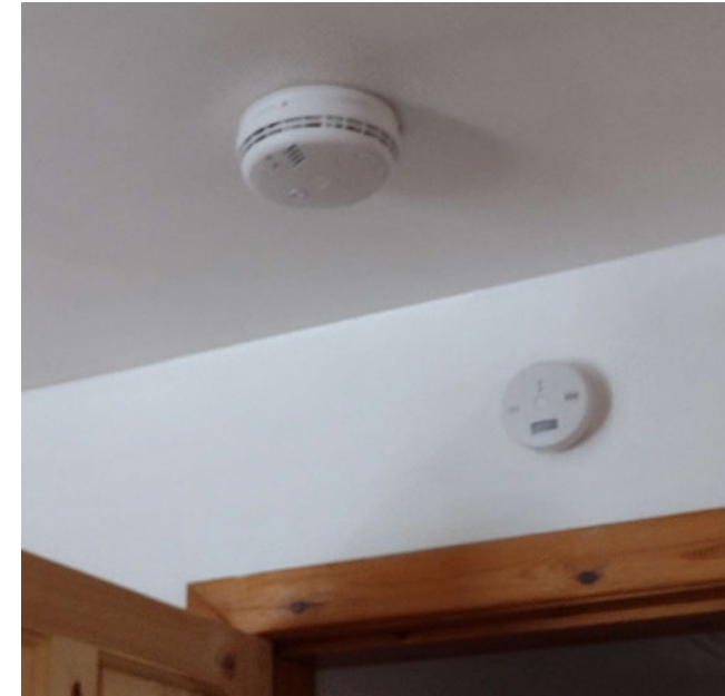
Smoke detector in living area
