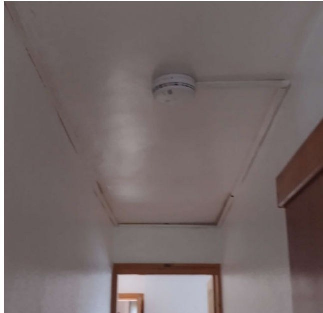
Smoke detector in hallway
