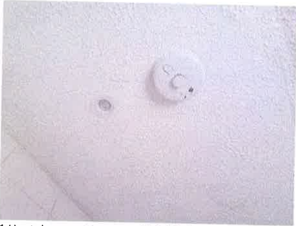
1 Heat detector present within Kitchen.
