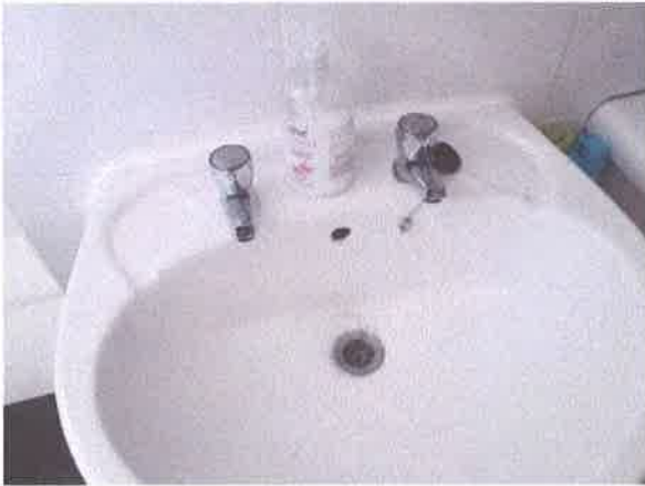
13 Wash basin – flow test.
