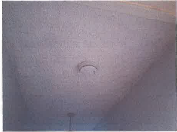
14 Smoke detector in Hall.
