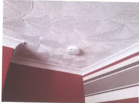
6 Smoke detector in Living Room.
