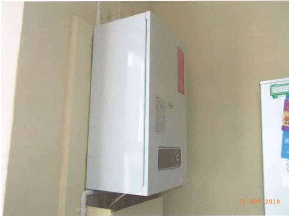
Central Heating Boiler
