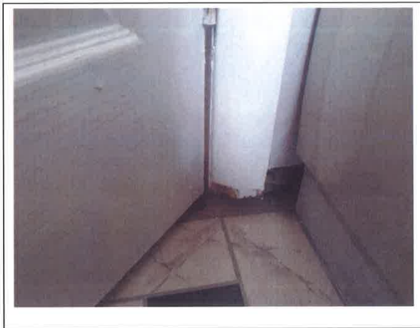
Rotten facing board within bathroom
